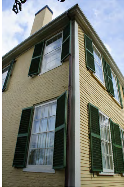
Figure 4: Transition from wood clapboard to brick at the southwest corner of building.
