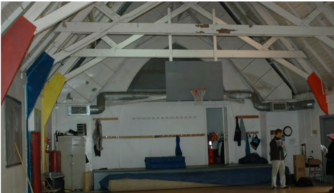
Figure 7: although now used as a gymnasium, vestiges of the original chapel can still be seen, including the open trusses, high ceiling, and the pointed arched opening at the apse.
