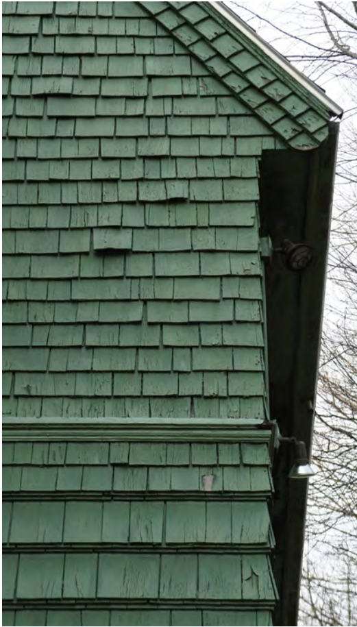
Figure 4: the shingle detailing was well-considered to create different effects at different parts of the building.
