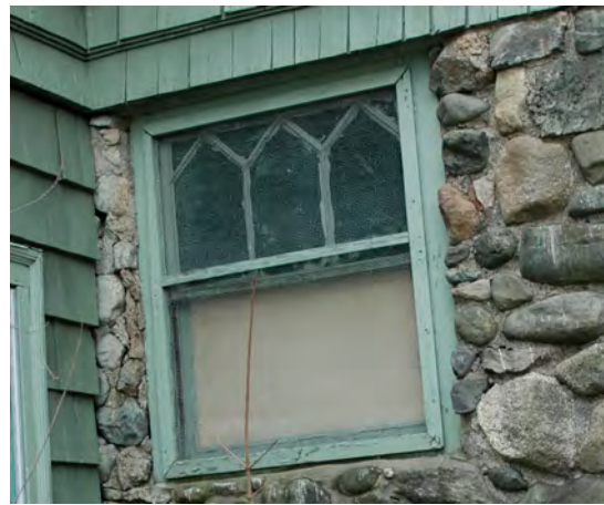
Figure 6: original windows with ornamental muntins still extant at lower level
