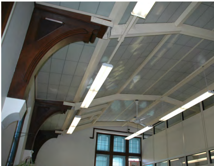
Figure 5 (left): (rotate/straighten and reinsert) original wood brackets on plaster corbels still extant. Inappropriate steel and Kalwall dropped ceiling obscures rest of trusses and ceiling
