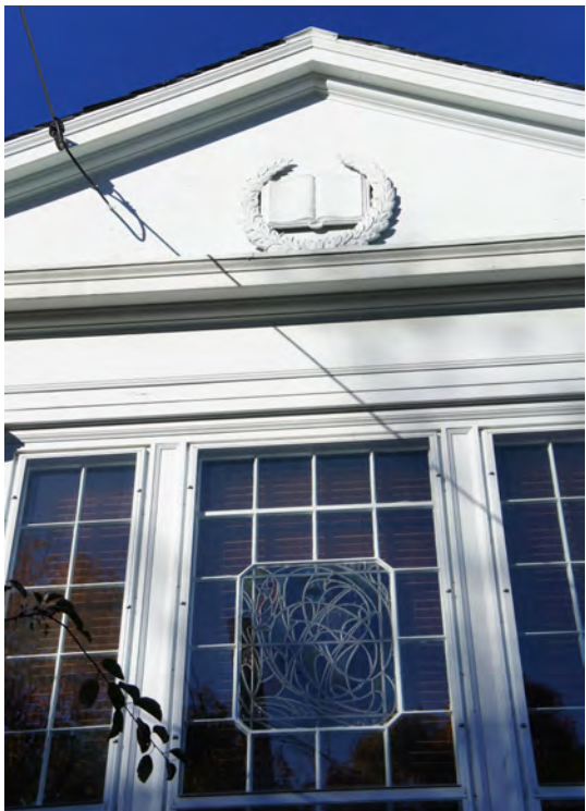
Figure 4: South gable end. Note carved pediment ornament and stained glass panel behind storm windows.
