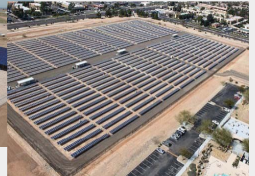
2 MW, Arizona State University
