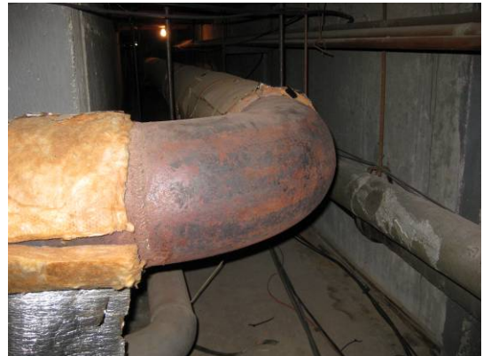
Exposed & Under-insulated Steam Piping
