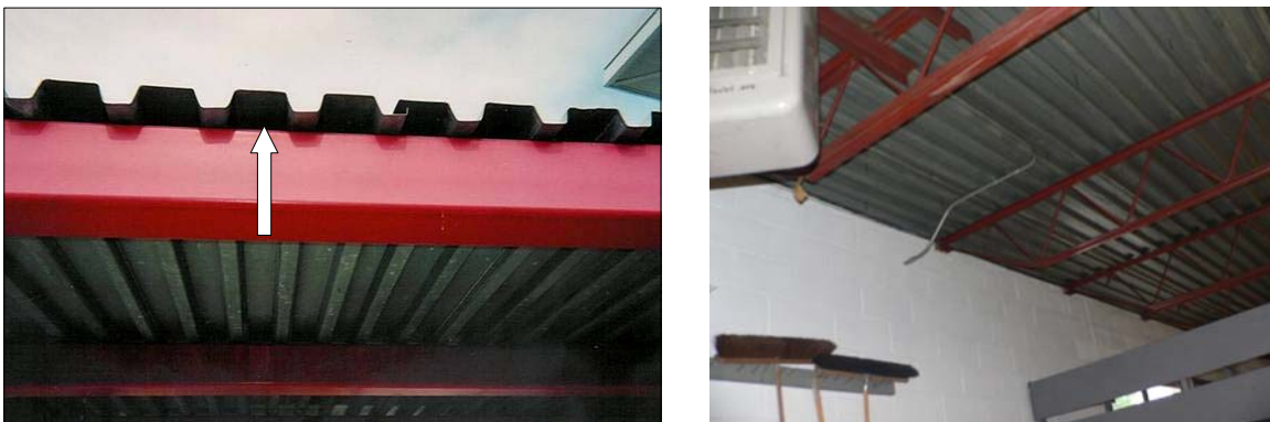
File Photos of roof panning (notice the gap between corrugations)
