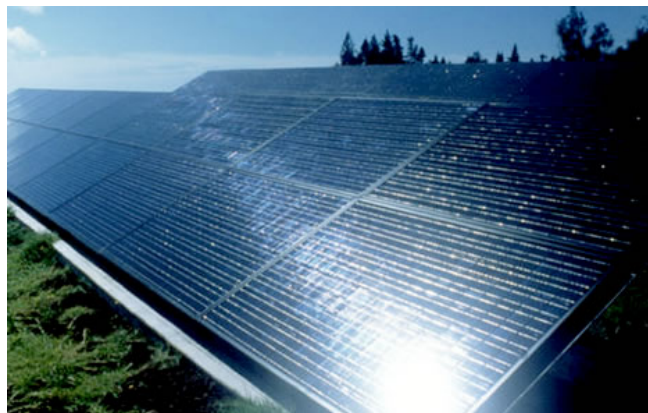
Solar PV Panel
