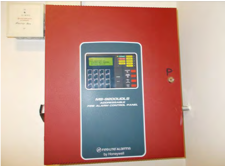
228 Webster Street Fire alarm panel
