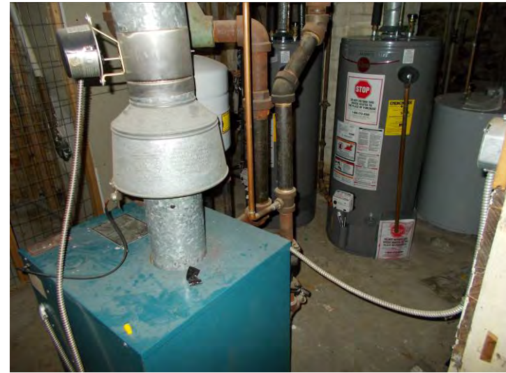
163 Jackson Road Typical Burnham boiler and Rheem domestic hot water tanks
