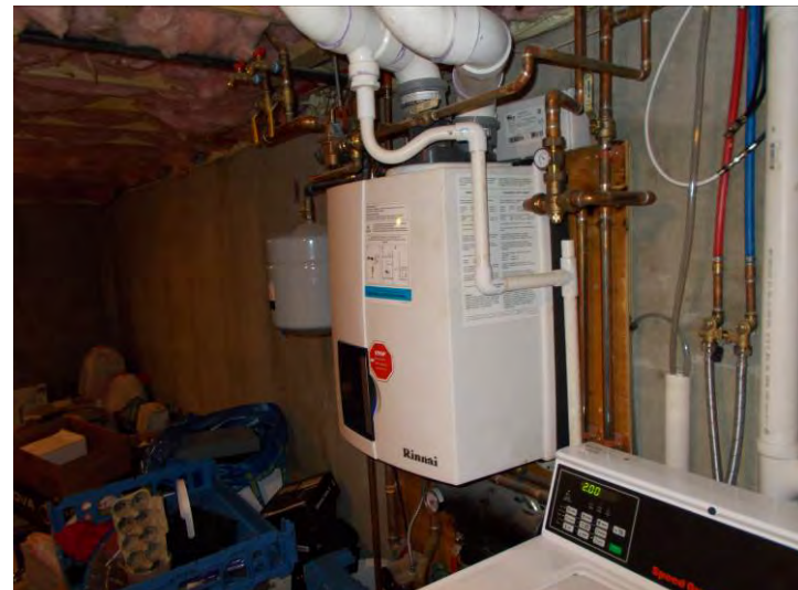
54 Taft Avenue Tankless domestic hot water system
