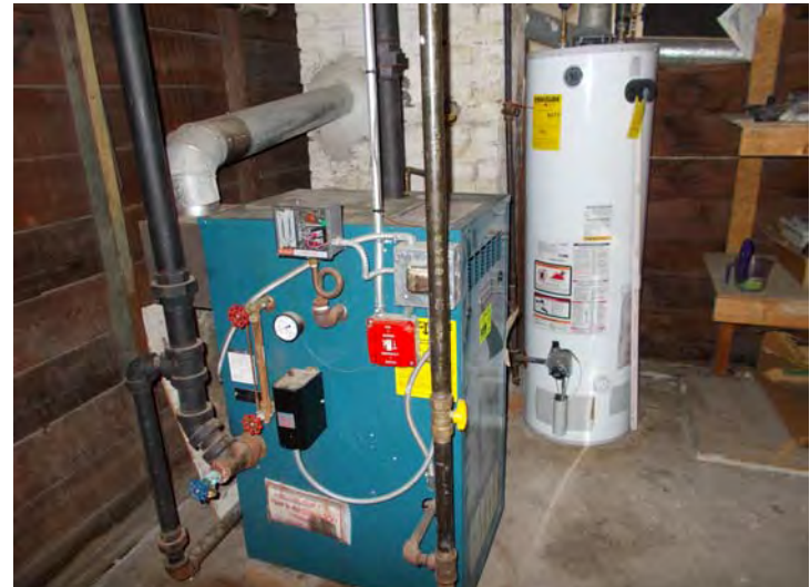
20-22 Falmouth Road Burnham boiler and Rheem 40-gallon domestic hot water tank
