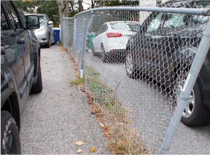
228 Webster Street Damaged fencing at driveway
