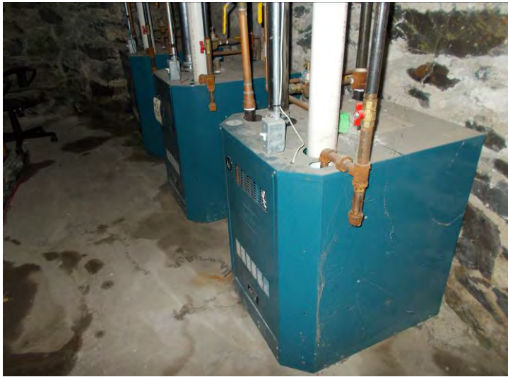
61 Pearl Street Burnham cast iron boiler for unit heat
