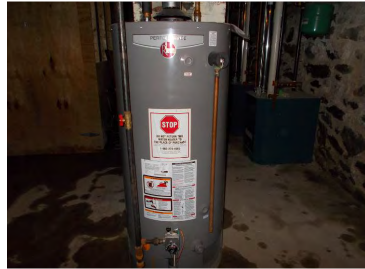
61 Pearl Street Rheem domestic hot water
