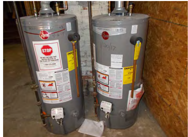
18-20 Cambria Road Rheem 40-gallon domestic hot water tanks
