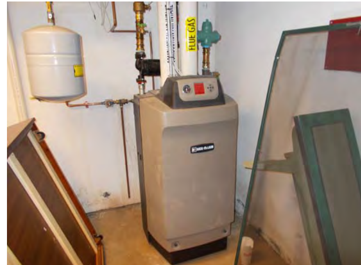
90 Christina Street Weil McLain boiler for unit heat for all units within the building
