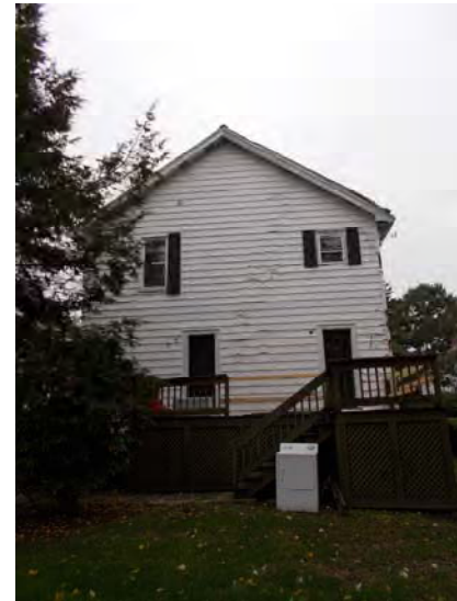
11-13 Cambria Road Rear façade damaged from fallen tree
