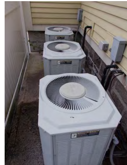
228 Webster Street Exterior condensing units
