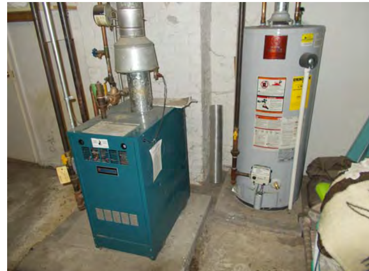
2148-2150 Commonwealth Avenue Typical Burnham boiler and Rheem 50 gallon DHW
