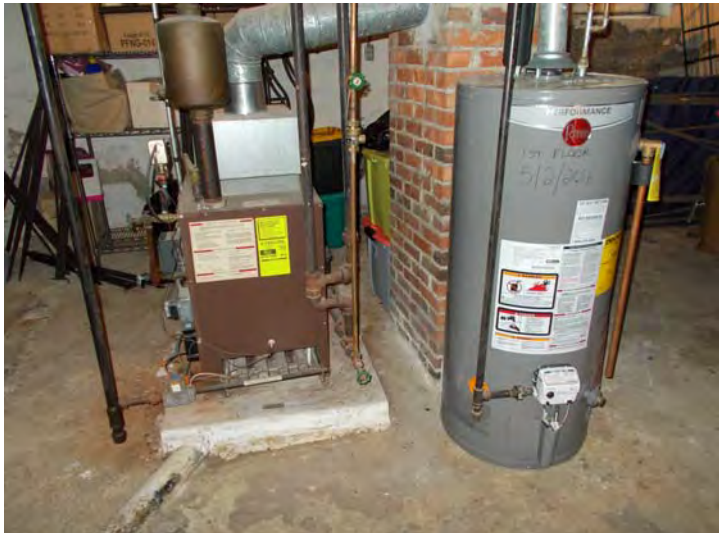
11-13 Cambria Road Typical of two boiler and domestic hot water tank
