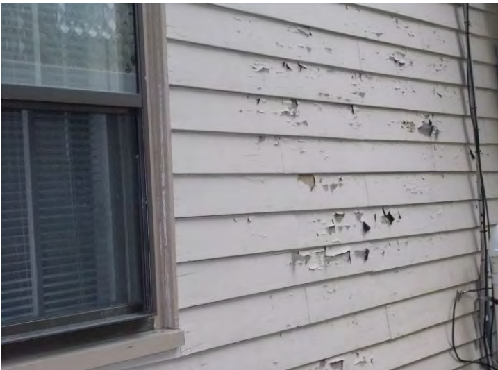
14 Nonantum Place Peeling paint and damaged wood siding
