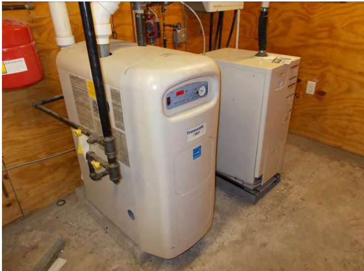
14 Nonantum Place Boiler and Cogeneration system installed in 2010
