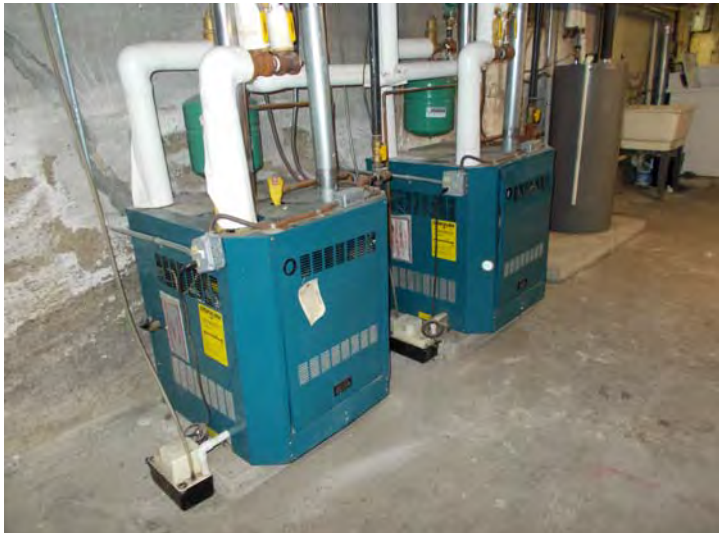
18-20 Cambria Road Burnham 96 MBH gas-fired boilers
