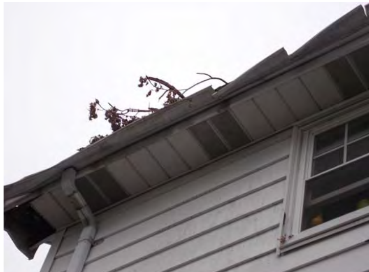
11-13 Cambria Road Roof damage from tree
