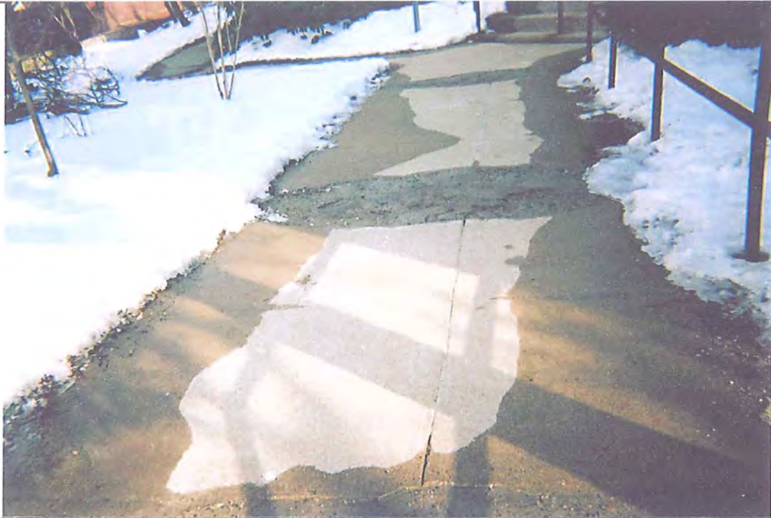
Deterioration of Sidewalk
