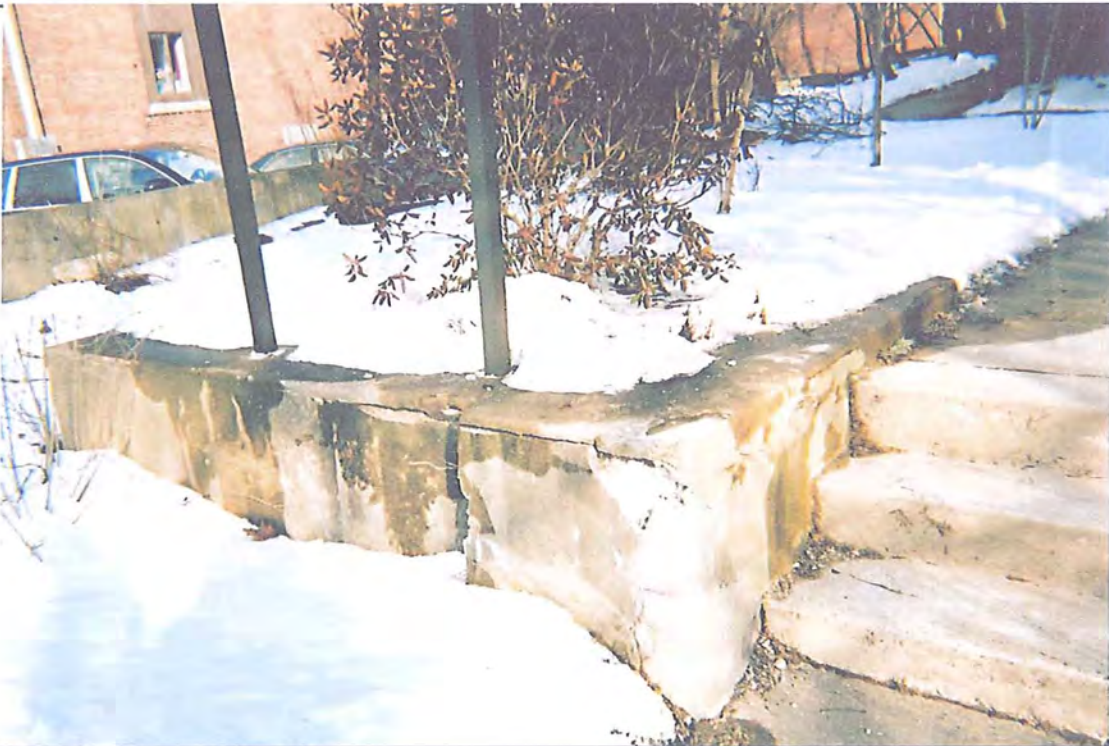
Deterioration of Concrete
