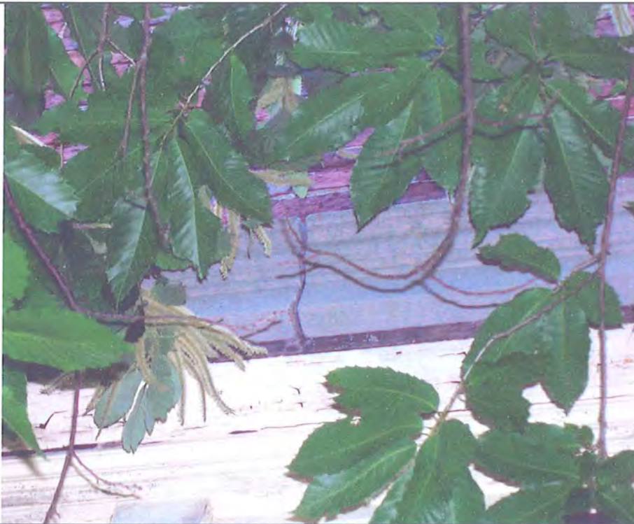
Crack in Stone Lintel above Window Type B-3
