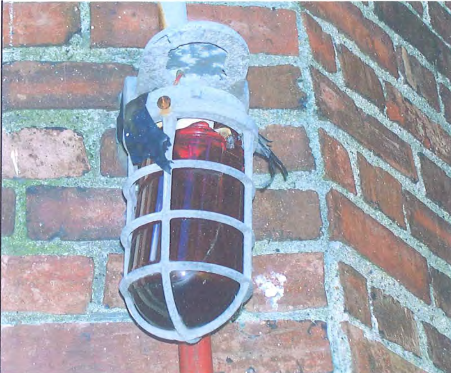
Broken Fire Alarm Beacon
