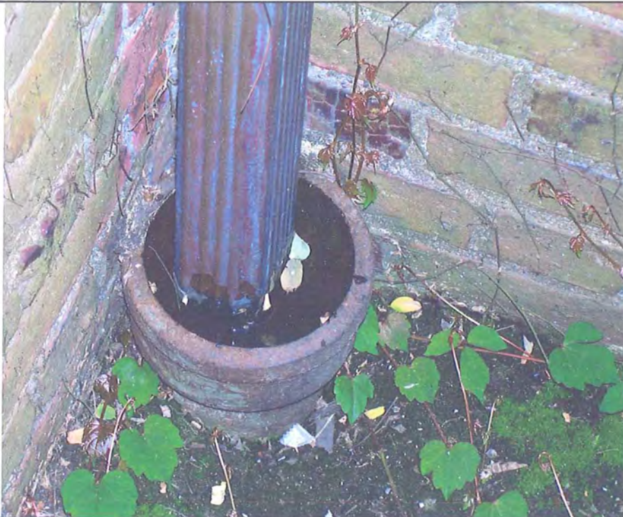
Blocked Vitrious Clay Drain Conduit
