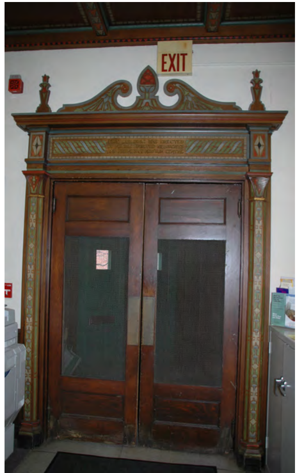
Figure 4: the ornamental wood architrave surrounding the pair of wood doors from the center room to the entry vestibule is stenciled in a multi-colored pattern. Note the wood ceiling above, which is similarly stenciled.
