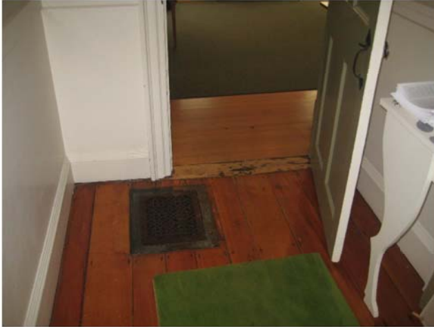
25. Typical Floor Grille on First Floor
