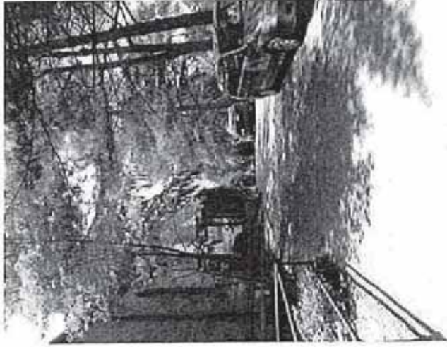
Figure 9: Driveway which needs to be repaved
