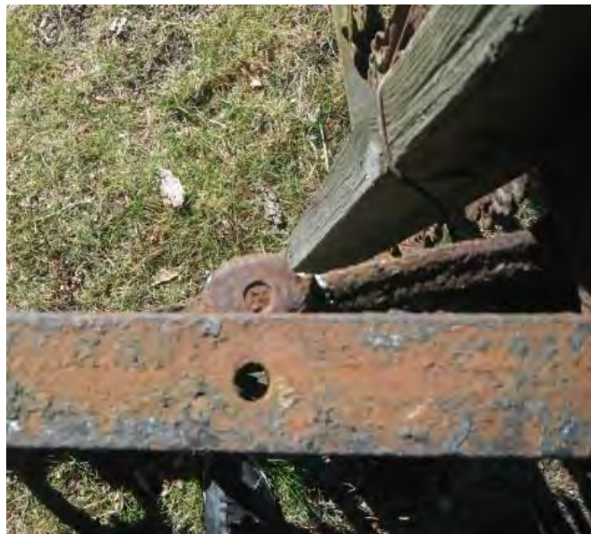
Detail: Degraded iron bolt which held medallion to the upper rail.
