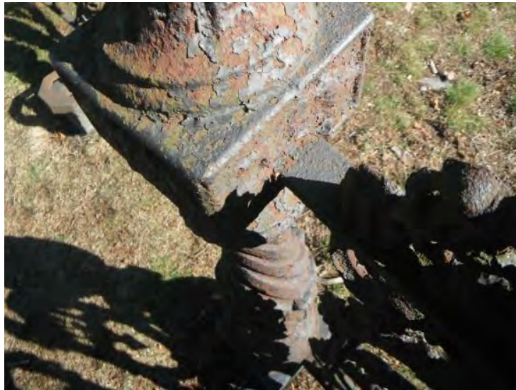
The iron is extremely corroded and rust covers at least 90% of the surface, which is pitted and still actively corroding.
