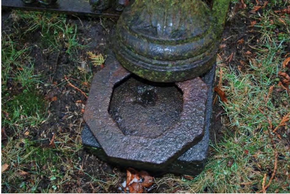
Detail: Corroded attachment of post to stone.
