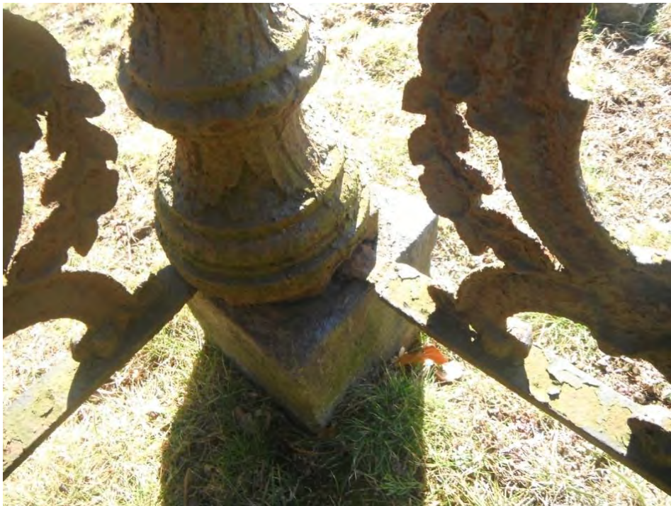
Detail: Corroded lower railing.
