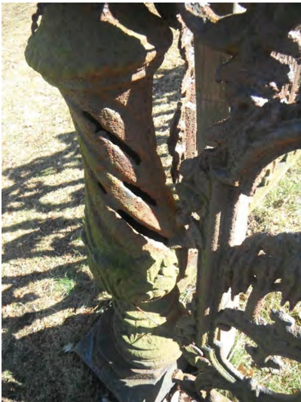
Several areas have corroded completely through and there is a significant amount of rust and loss of detail on the lower portions of the posts, medallions and lower rails.
