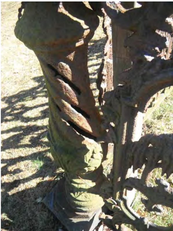
Several areas have corroded completely through and there is a significant amount of rust and loss of detail on the lower portions of the posts, medallions and lower rails.
