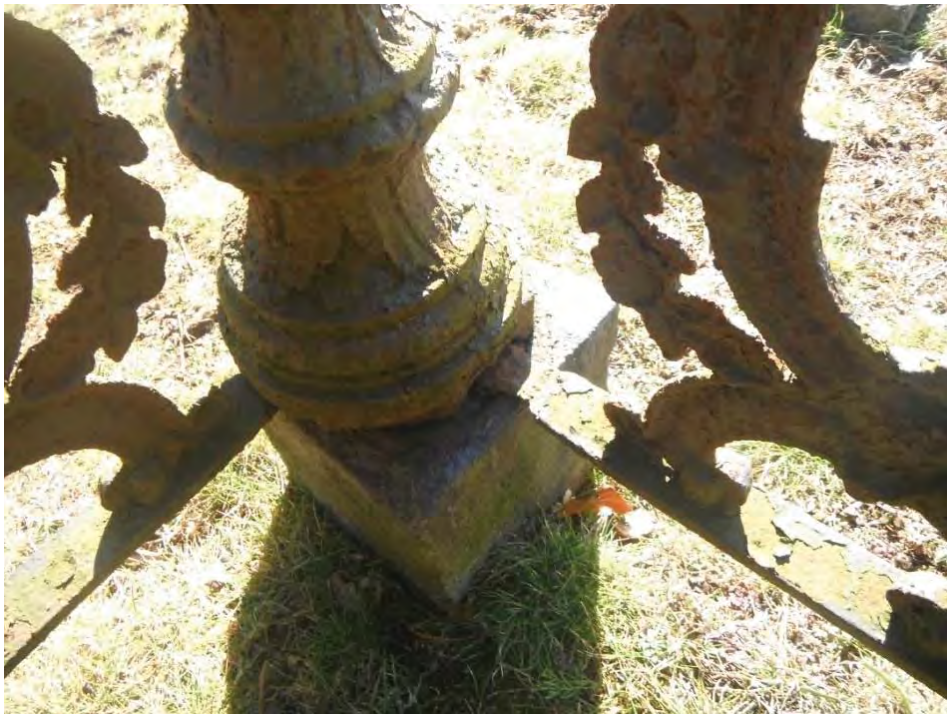
Detail: Corroded lower railing.
