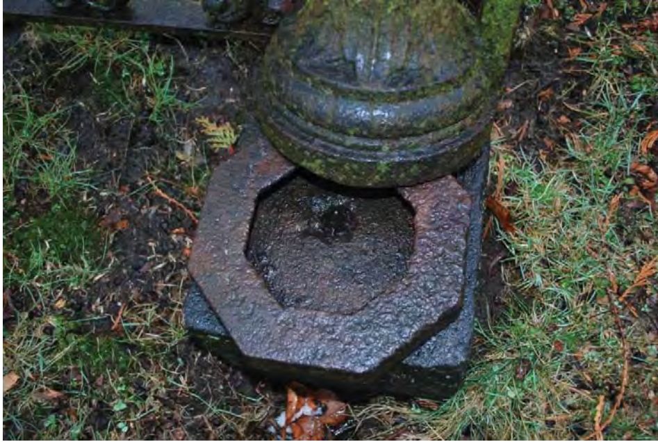
Detail: Corroded attachment of post to stone.
