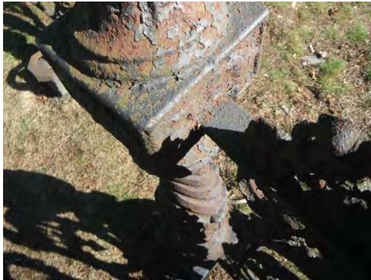
The iron is extremely corroded and rust covers at least 90% of the surface, which is pitted and still actively corroding.
