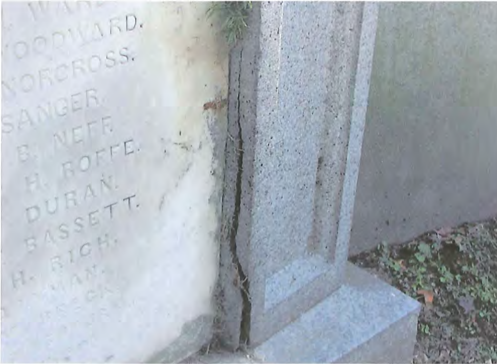
Photo D - Stress Crack in Granite Post & Staining of Marble Tablet
