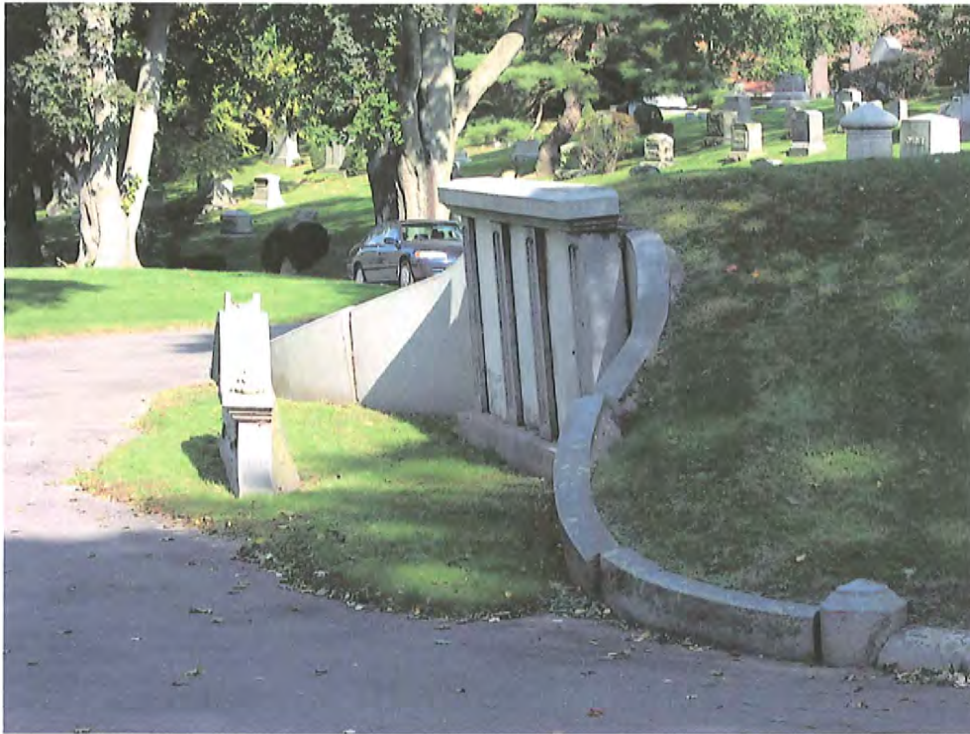
Photo C - Overall Photo of Curved Retaining Wall Showing Tilt of Central Portion, Displacement of Curved Stones & Cartouche from Top of Monument on Ground in Front of Monument
