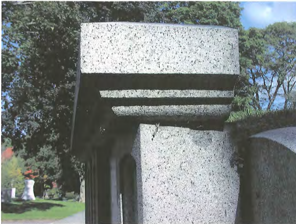
Photo E - Twisting of Posts and Displacement of Cap
