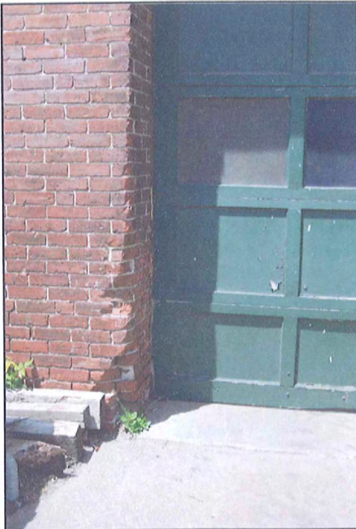
Garage Door at Basement - Damaged Brick Jambs
