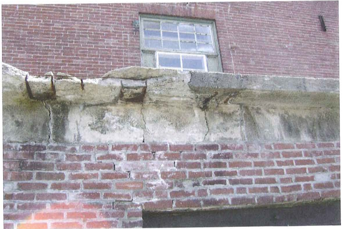
Photograph #18 – View of deteriorated concrete deck and step crack in brick walls below the deck.
