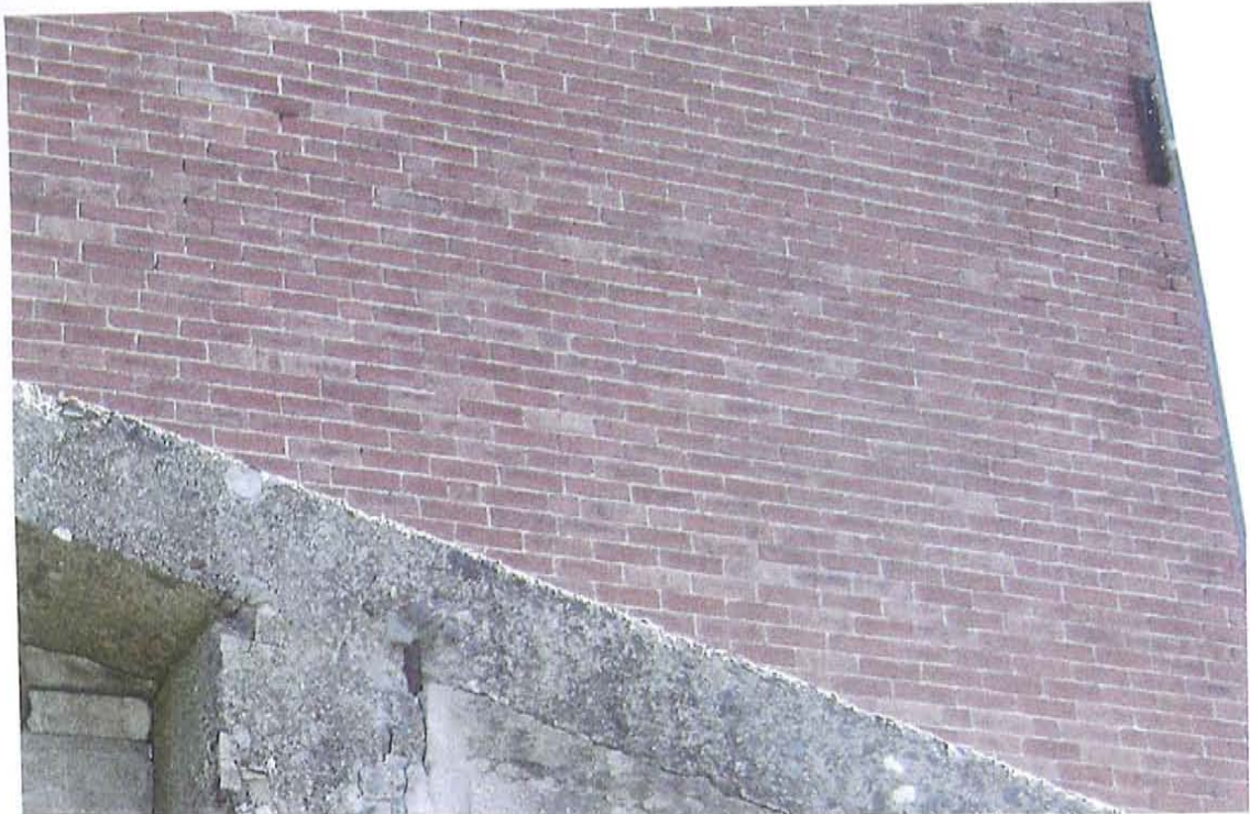
Photograph #17 – View of voids in the mortar joints in the rear brick walls.
