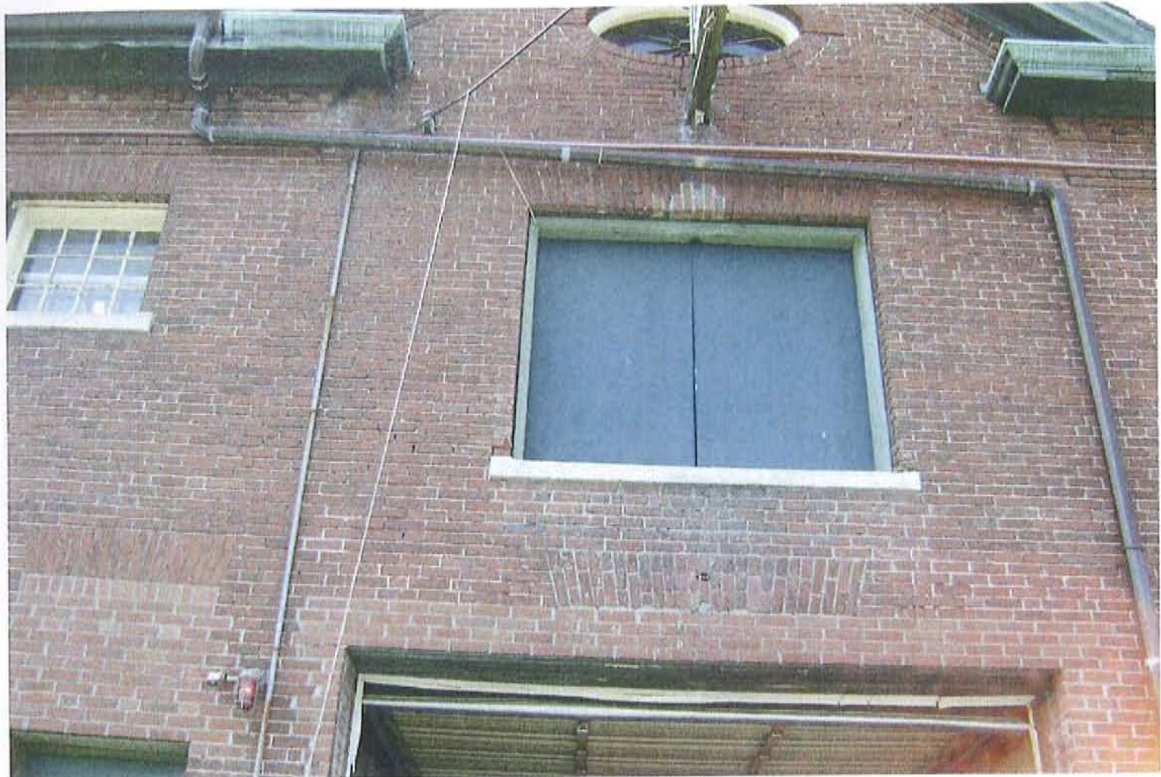
Photograph #15 – View of void in head joints, weathered back mortar joints, and holes in the brick wall where fixtures have been removed.
