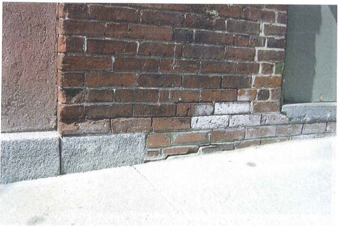
Photograph #16 – View of spalled brick, weathered back mortar joints, and crack between stucco infill and the brick wall
