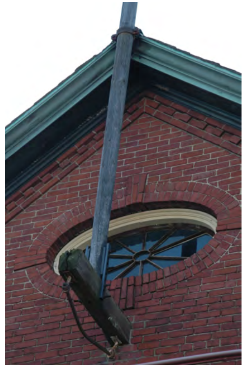
Figure 5: Oval window in brick frame at gable end. Note ornamental dentil brickwork at eave.
