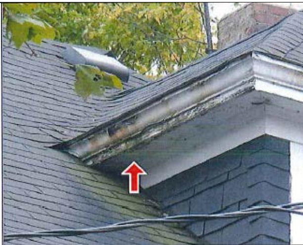
Rotting wood at dormer
