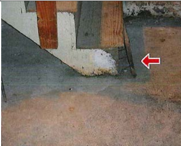
Rotted wood at basement stairs
