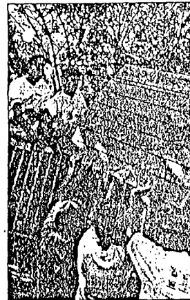
Left, Peter Budhish and Bruce Nelson worked with a crowd of volunteers to put up a roof at the newly revitalized playground.
