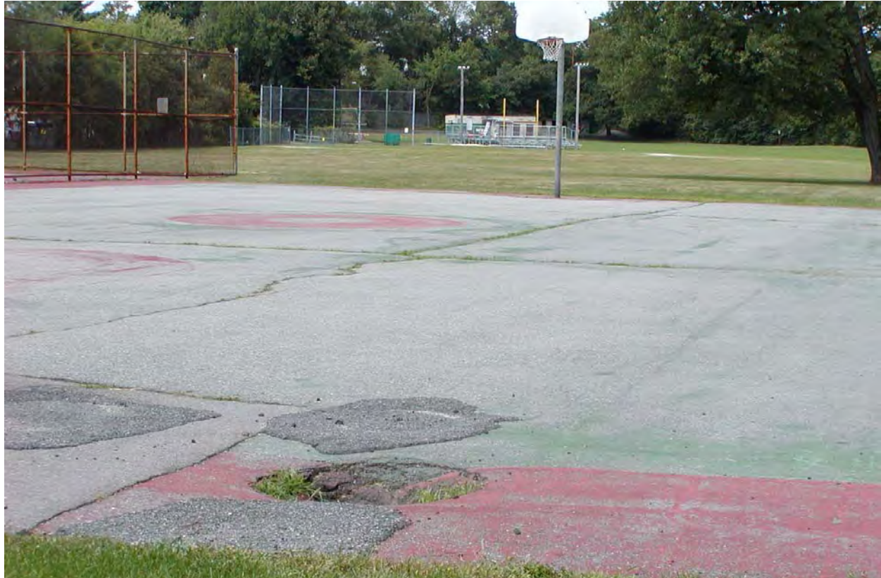
The basketball court is located in close proximity to Dedham Street. Deteriorated conditions (pavement settlement exhibited above occurs above an existing storm drainage culvert) make play difficult and unsafe.
