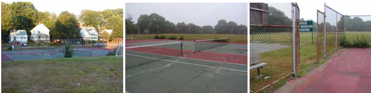
The tennis courts possess major structural deficiencies.
