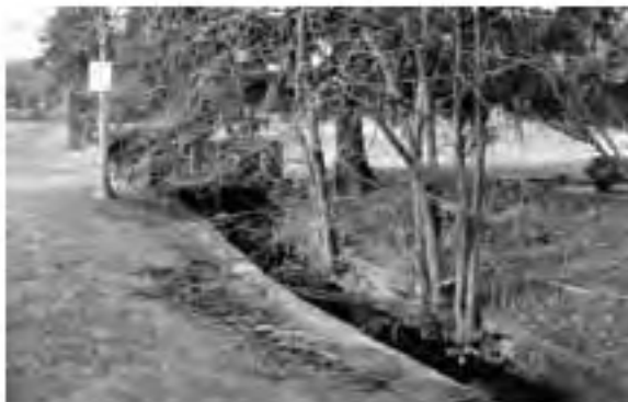
Volunteer trees growing in Hammond Brook channel walls, 2006
