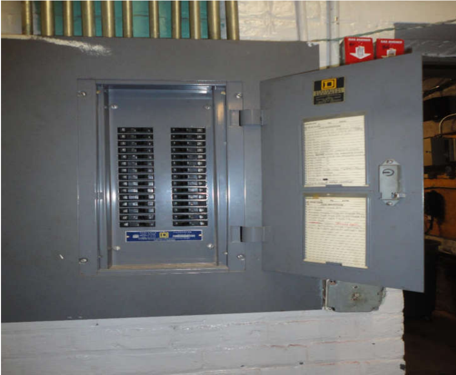
Photograph No. E-03 Upgraded Square D load center in basement
