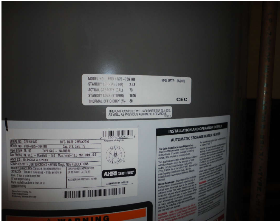
Photograph No. P-02 RUUD domestic hot water heater (2016 installation)
