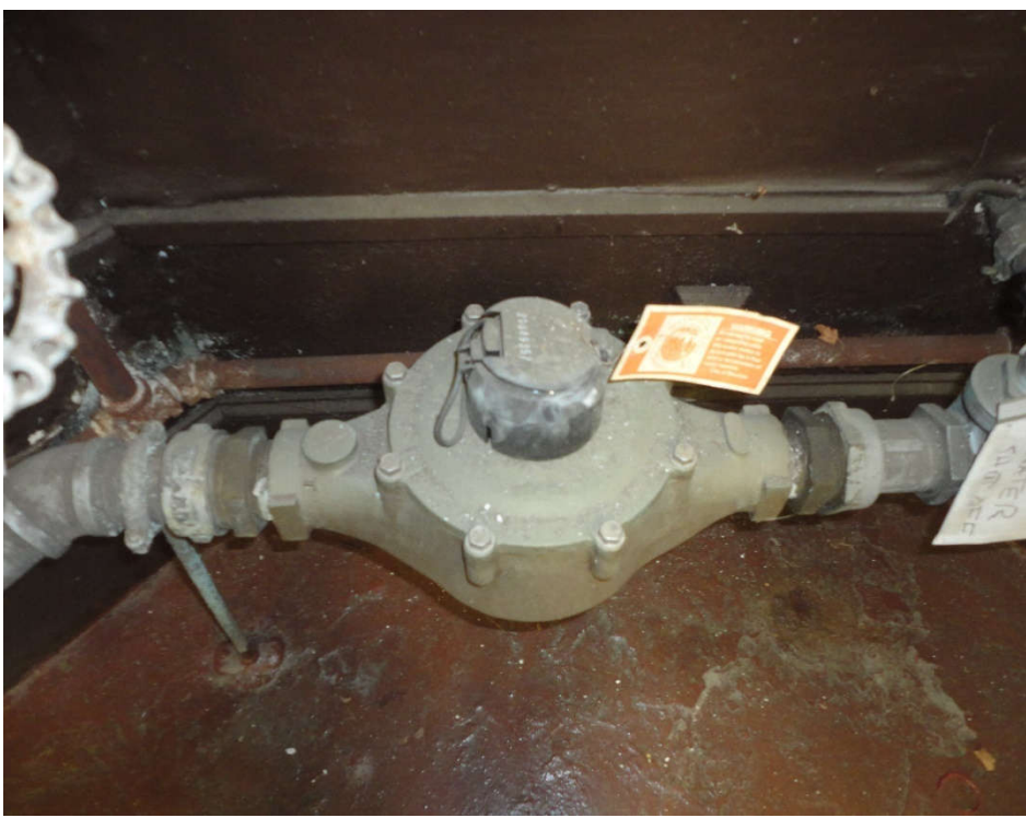
Photograph No. P-01 Incoming 2.5-inch water service and meter
