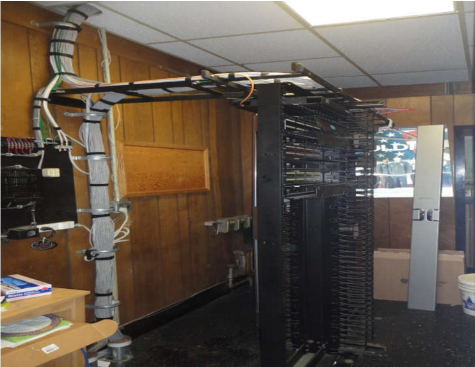
Photograph No. E-04 Main telephone-data service and server rack
