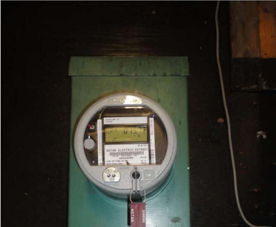
Photograph No. E-01
