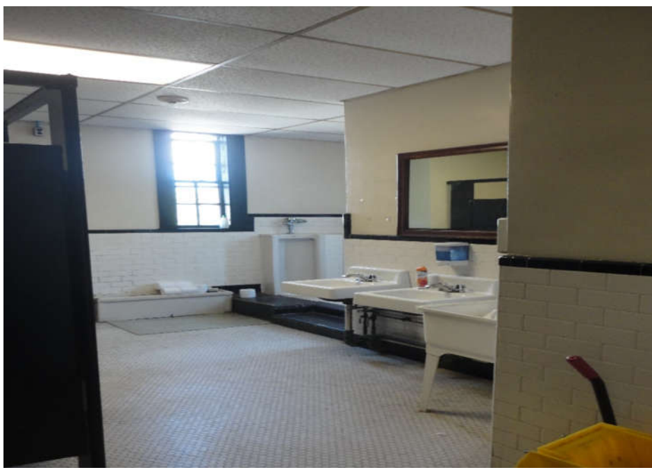
Photograph No. P-03 Representative plumbing fixtures largely original to the building
