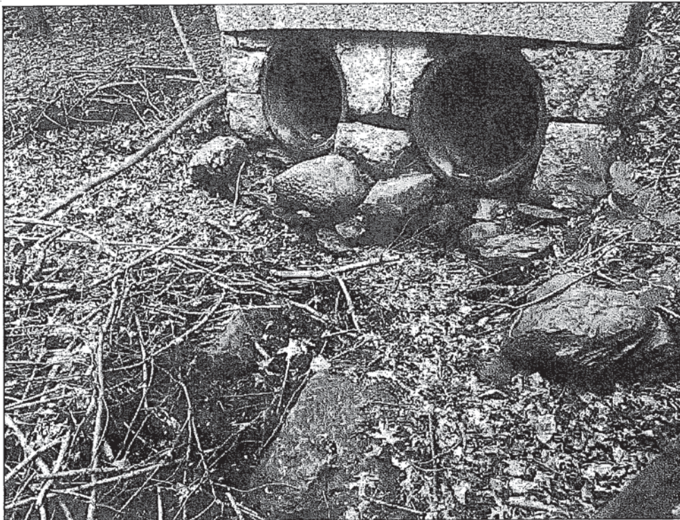
Photo No. 12: Low level outlet discharge headwall and standing water in the downstream channel.
