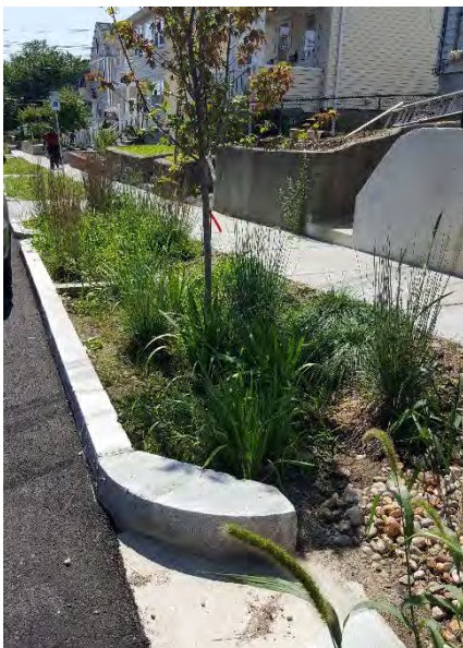
Bioretention Curb Bump-out Edenfield Ave, Watertown
