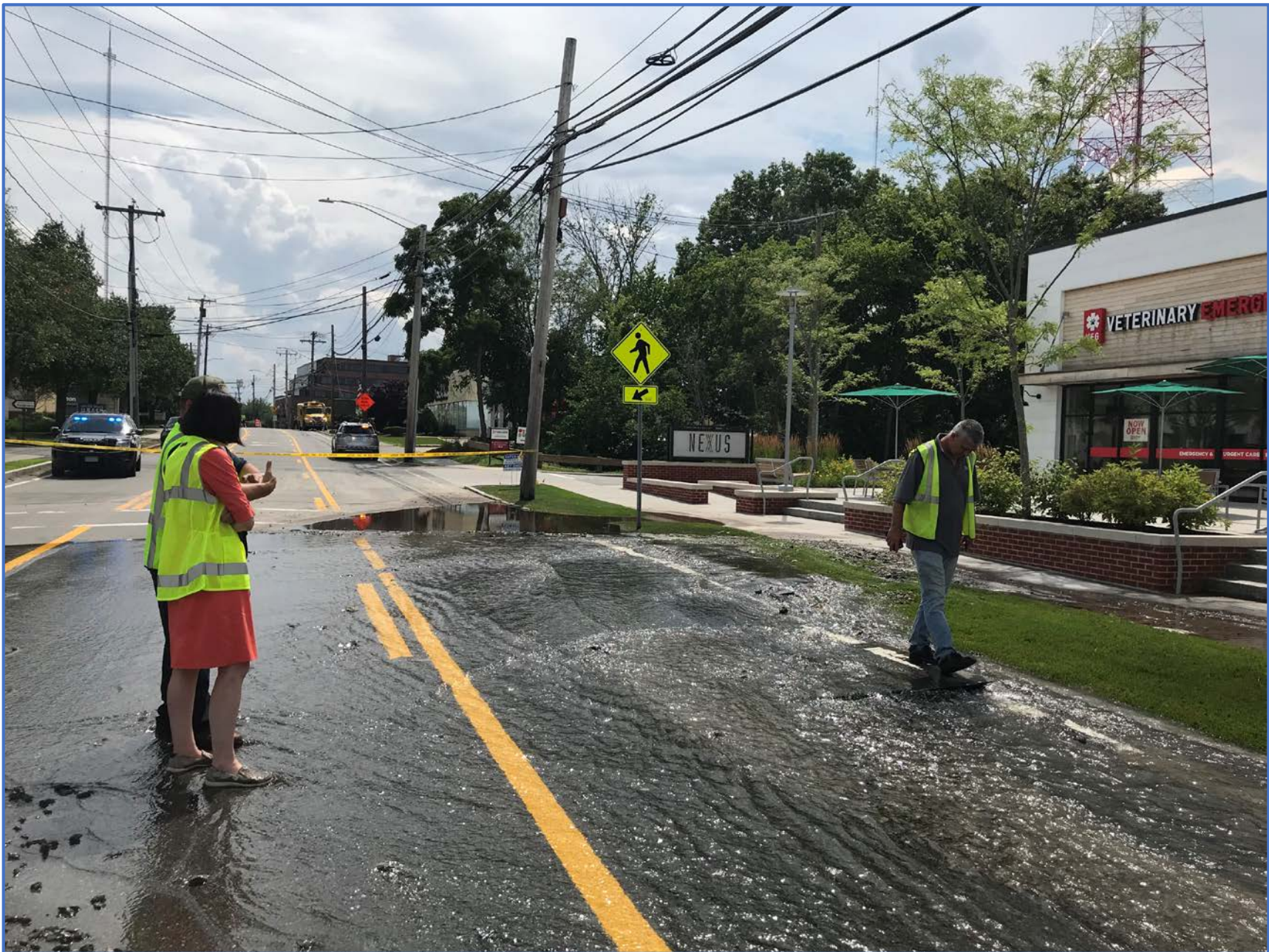
Needham Street Water Line Break, July 17, 2019
