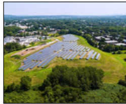
Renewable Energy: Solar array at Rumford Avenue
