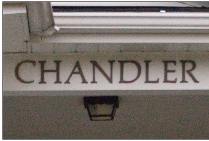
Simple signs, such as these individual letters on a historic building in Auburndale, can accomplish the goal of signage without compromising the historic building.
