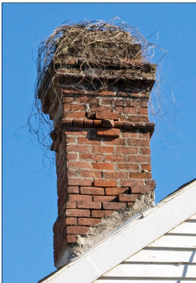
This chimney is leaning and has several visible open joints. Rebuilding to match existing detailing is recommended.
