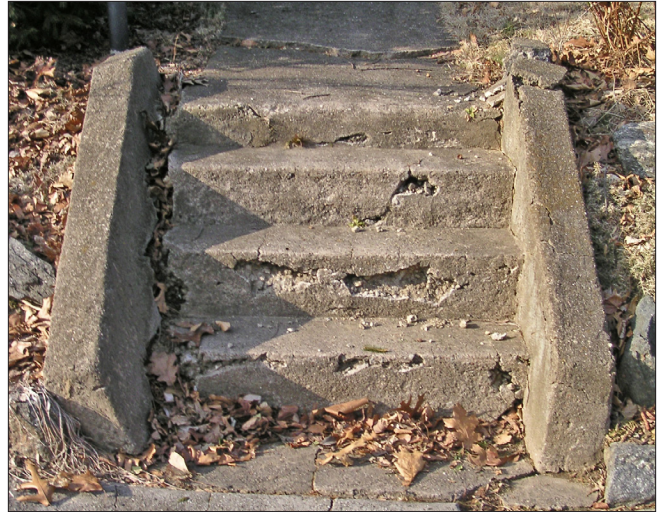
Without proper upkeep, tripping hazards can develop at steps and walkways. There are significant cracks and openings at these steps, exposing the reinforcing bars to stormwater and de-icing salts. This can accelerate the rusting of the reinforcing and deterioration of the concrete.
