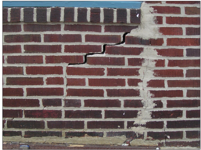
A previous vertical crack has been improperly repaired with hard grout smeared onto the wall surface. The second diagonal crack suggests a settlement or movement problem, that warrants consultation with an architect or engineer.
