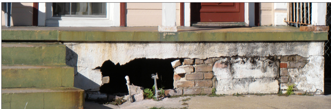
The stucco has not been maintained and the bricks under the porch post are falling out of position. The dislodged bricks can lead to structural problems in the porch if not repaired.
