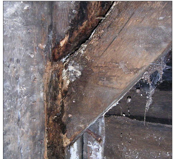
The dark areas at the top and side of the diagonal wood brace indicate moisture. The end of the diagonal wood frame is rotting. The cause of the moisture infiltration should be addressed and the wood framing repaired.
