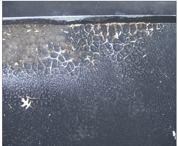
The alligatored roof surface indicates deterioration and possible need for replacement.
