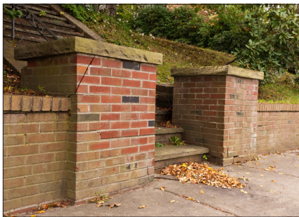
Similar to building walls, landscape walls and fences require regular maintenance, particularly at retaining walls. There is significant cracking at both of the piers that might indicate a structural problem.
