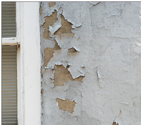
The peeling paint is likely incompatible with the stucco or caused by moisture. Loose and flaking paint should be removed and peeling cause determined before repainting.
