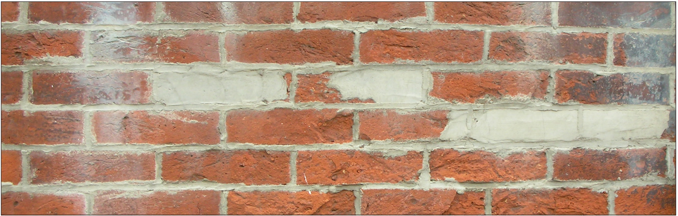
The rough texture and uneven surface suggest that an overly aggressive cleaning method was used. Stucco patches replace bricks and efflorescence, a powdery white substance, can be seen on the surface.
