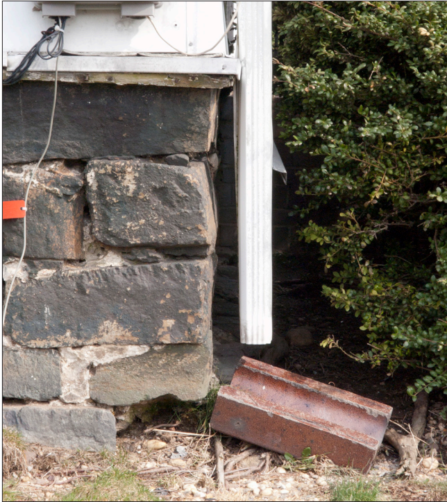
The storm water from the downspout has deteriorated the foundation's mortar and the bottom stone has been dislodged. It is recommended that water from the downspout be directed at least 3 feet away from the foundation and that the shrubs be trimmed or relocated away from the building.
