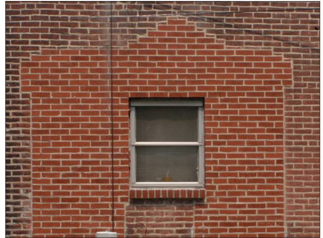
The brick infill area is clearly visible. The infill area uses bricks of a different size and color than the historic bricks and is outlined by a thicker mortar joint rather than being "keyed" into the adjacent brickwork. The bricks and mortar used in the infill areas should be the same size, color, texture, appearance, profile and hardness as the adjacent historic bricks. The repair should also be "toothed" into the adjacent brick to appear continuous with the wall surface.
