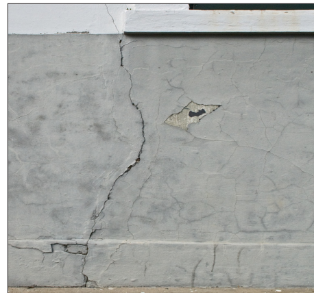
The crack from the window sill might be a sign of building settlement. Review wall for other signs of movement or settlement. Repair crack and apply a lime-based paint for a uniform appearance.
