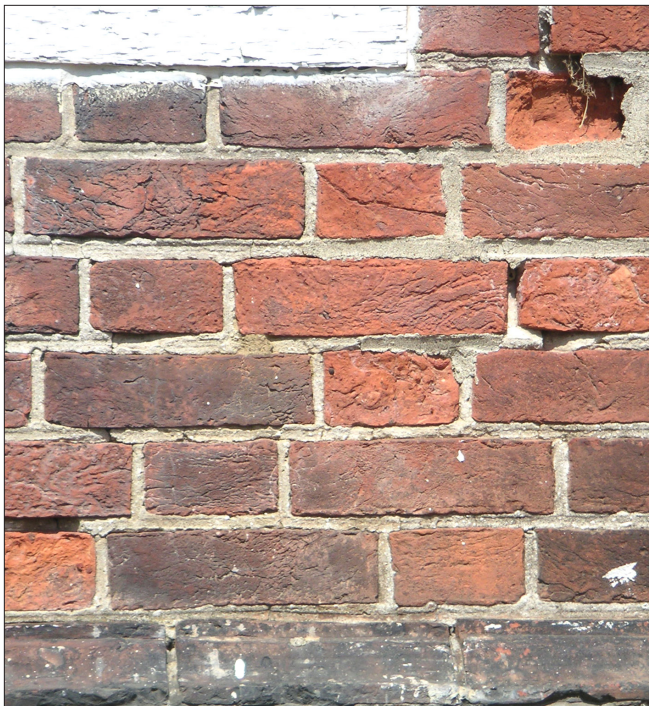
The repointing mortar in this wall is likely harder than the bricks, containing too much Portland cement. The surface of the upper brick has spalled, exposing the softer interior of the core. The mortar is also beginning to crack and pop out of the lower joints.
