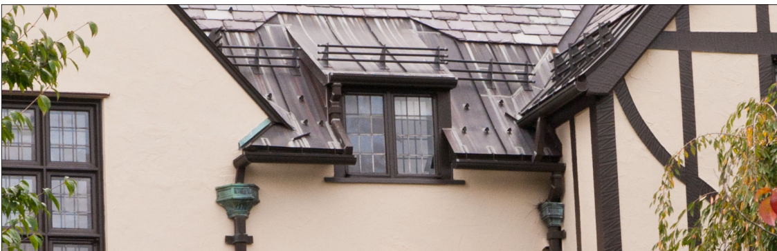
Snow guards come in a variety of types and styles, as seen on this roof. Also note the standing-seam metal roof with copper gutters, downspouts and decorative copper scuppers.
