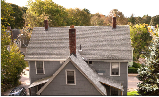
Asphalt shingles are a common 20th century building material, for both roof replacement and new construction.
