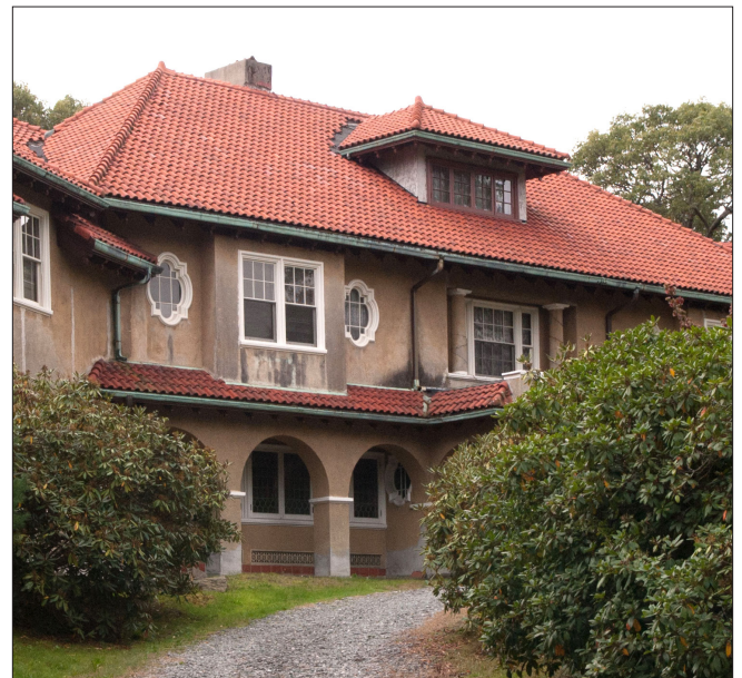
Tile roofs can often last as long as slate roofs, and contribute greatly to the character of buildings such as this historic home.
