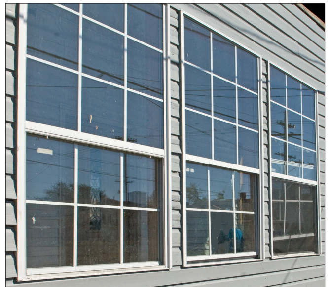
The 9-over-6 vinyl replacement windows have applied muntins, are mounted flush against the outside wall and lack the depth of traditional windows. They do not have trim or casings. They are not appropriate for historic buildings.
