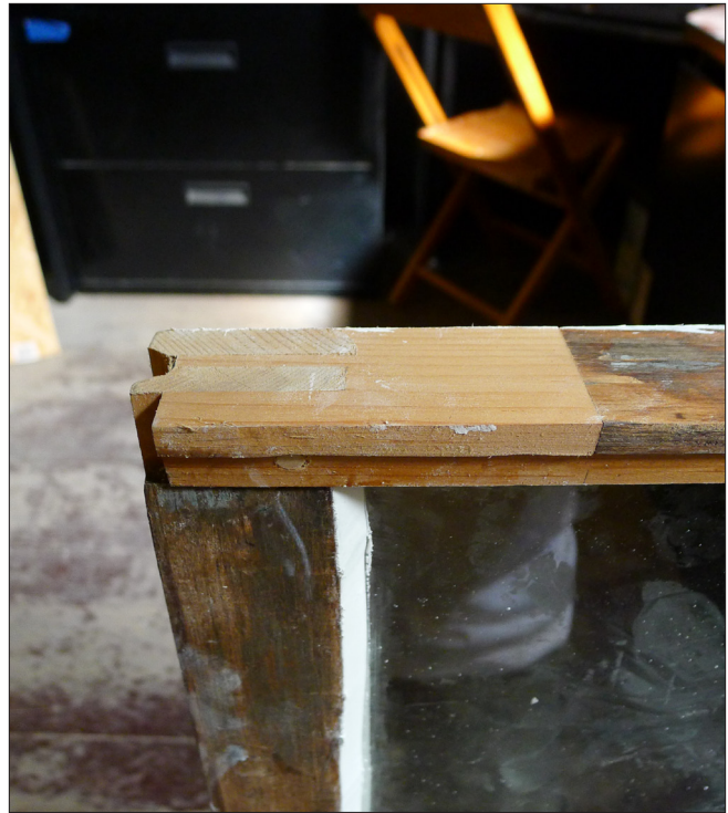
One of the advantages of historic wood windows over modern prefabricated units is repairability. This photo demonstrates a dutchman repair at the corner of a historic wood window. Also note the new glazing putty.
