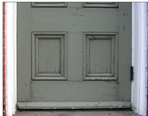
Wood checking and peeling paint is visible. Minor repair and maintenance can prolong the serviceable life of this door.
