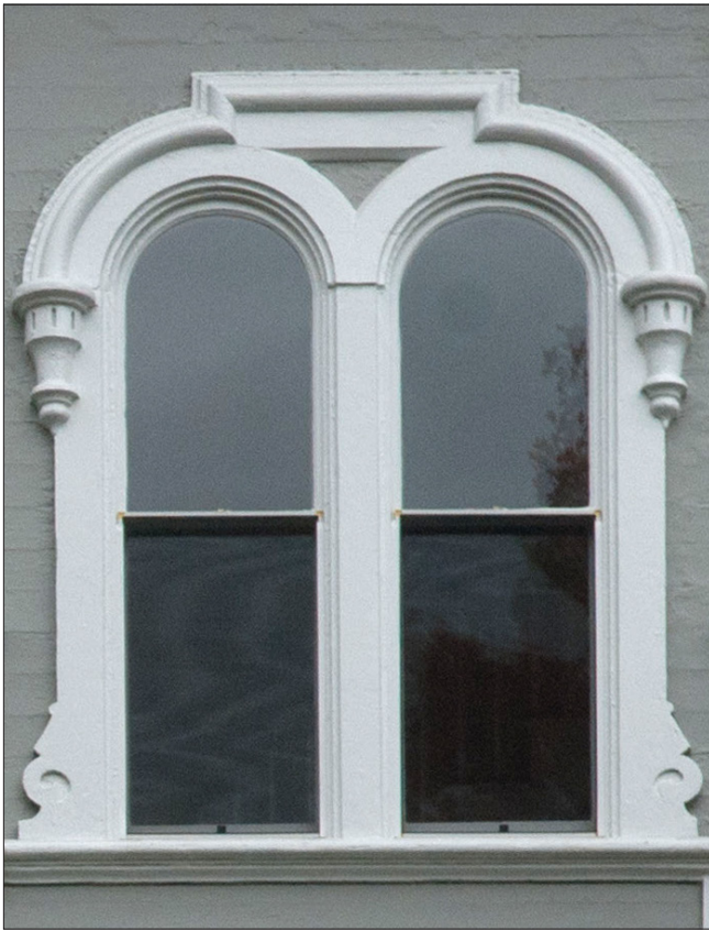
The highly ornate trim surrounding this paired, round-headed, Italianate window is a significant feature that should be maintained. The installation of replacement windows often requires the installation of a new frame that can damage or visually alter the relationship between a window and its historic surround. Care should be taken if window replacement is considered.
