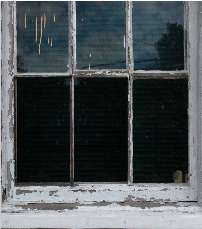
Typically, the deterioration of wood windows first occurs at the sill. Peeling paint can allow moisture to enter wood and cause rot. Regular repainting is recommended to provide a protective layer against moisture.
