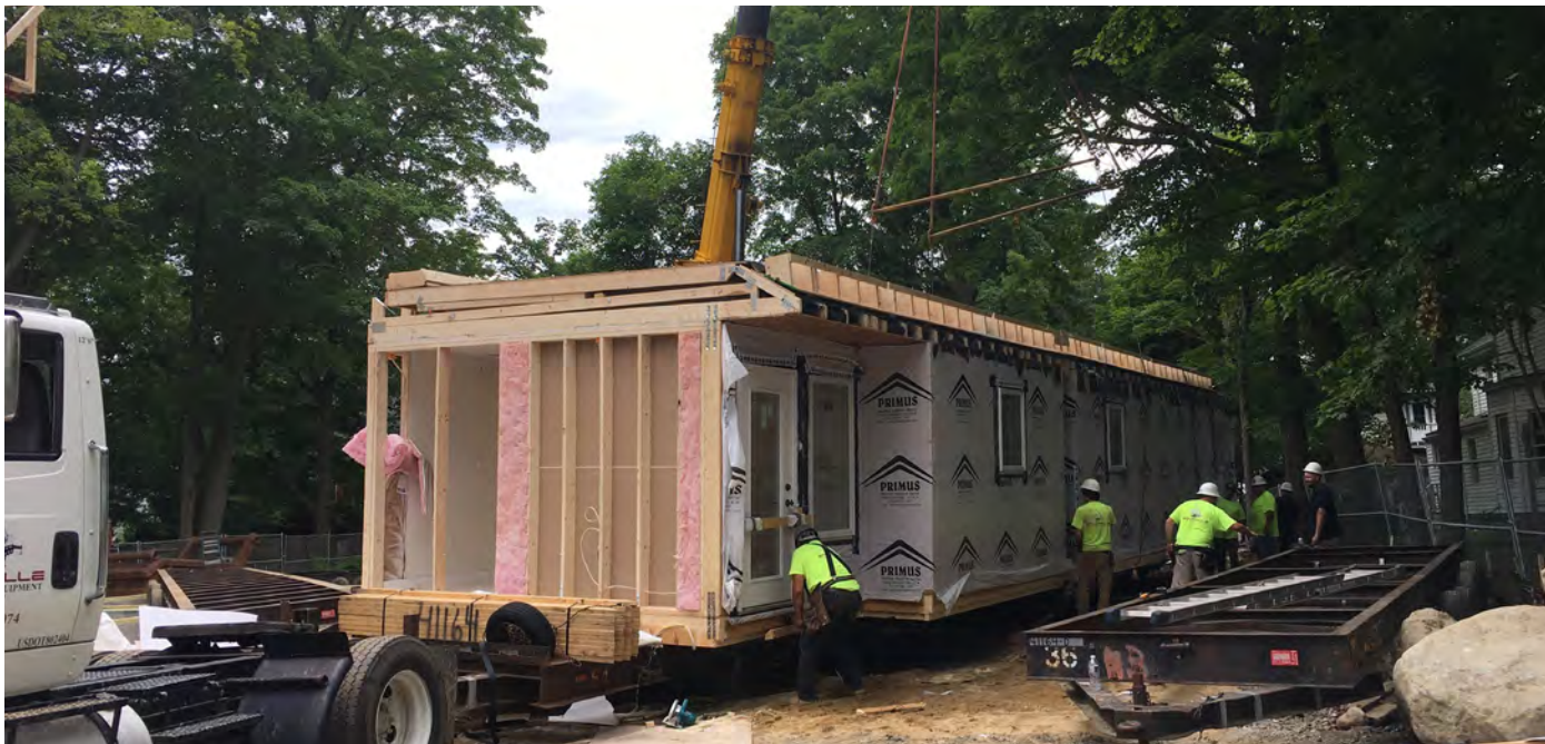
New affordable housing under construction on Auburn Street, a project supported by funds from Newton's housing programs.
