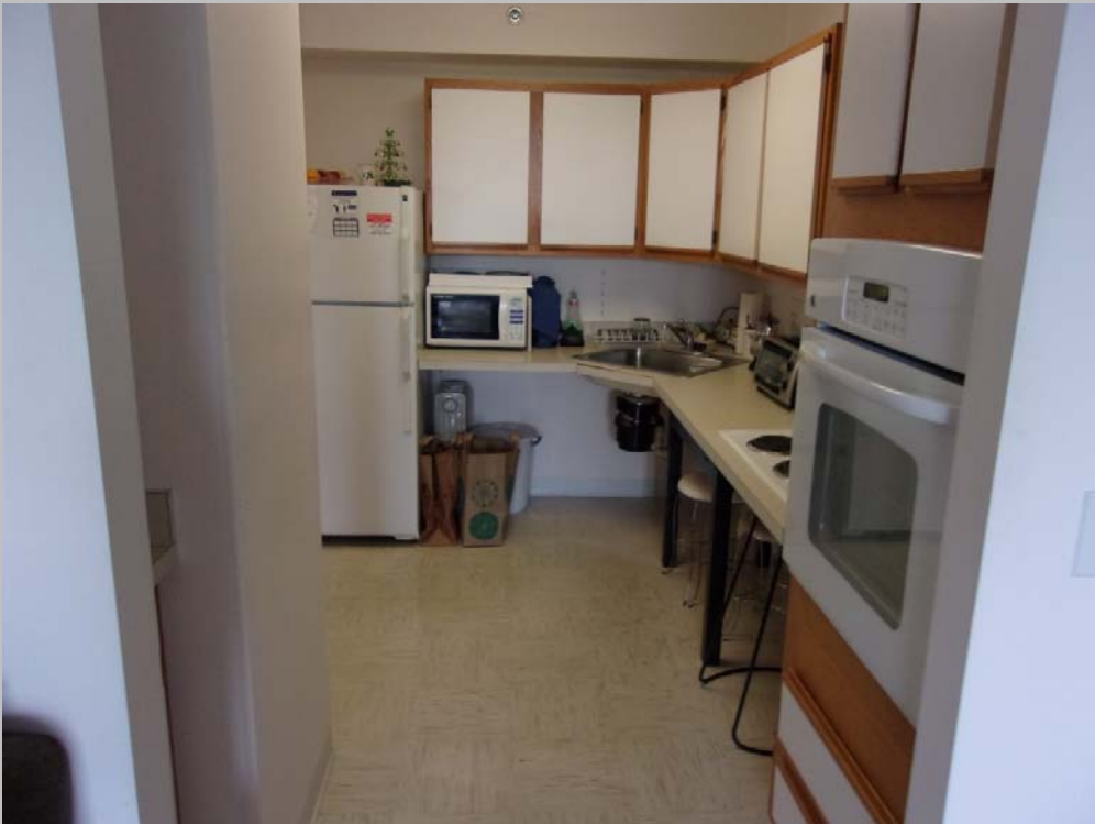
Coleman II handicap dwelling unit without scald and abrasion protection under sink (Critical Repairs)
