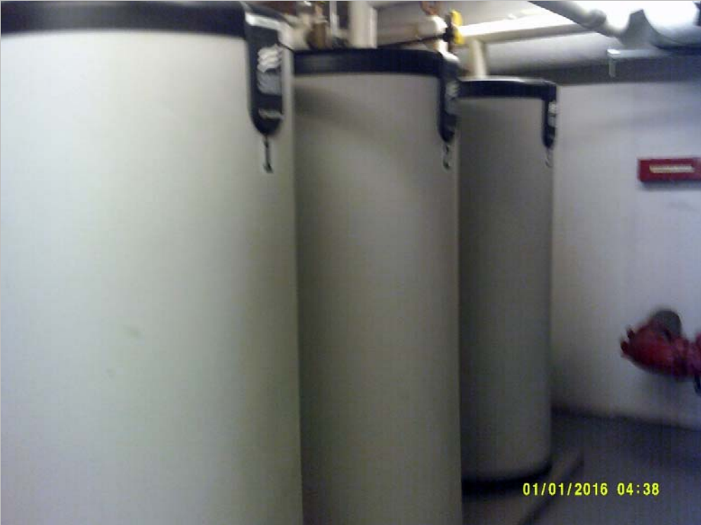
Hot water storage tanks
