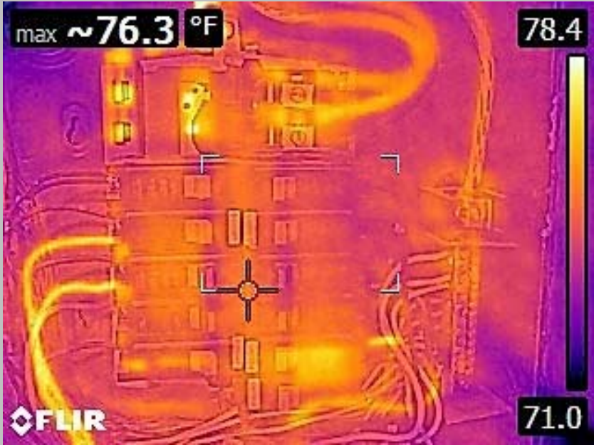
Thermal Image of Dwelling Unit Breaker Panel with Low Temperature Reading
