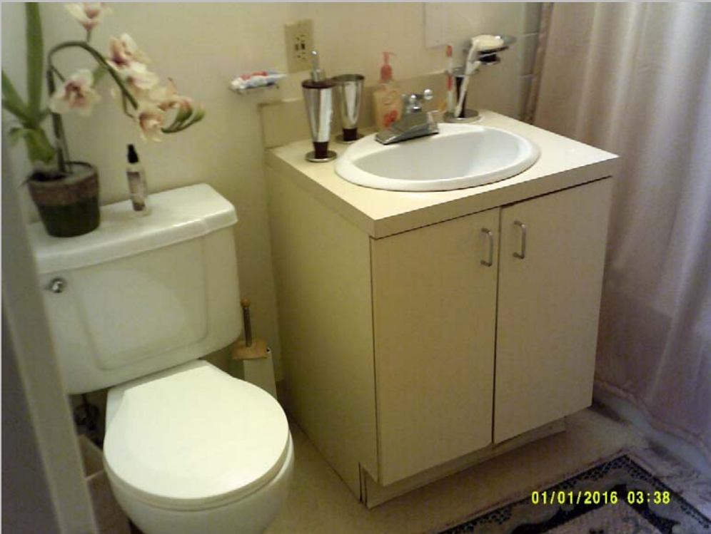
Standard dwelling unit bathroom in Coleman I with GFCI outlet
