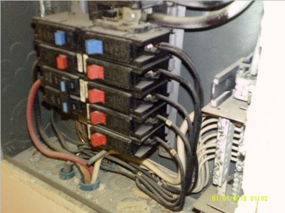
Top right breaker double tapped in Coleman I dwelling unit (Critical Repair)
