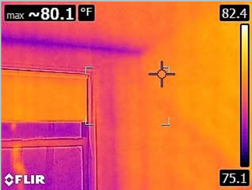
Thermal Image of Dwelling Unit Exterior Wall, Window, And Ceiling Without any Moisture Detected
