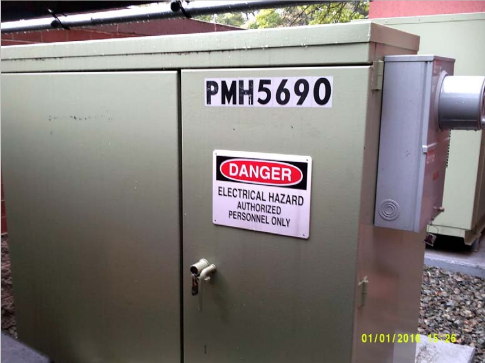
Pad mounted transformer
