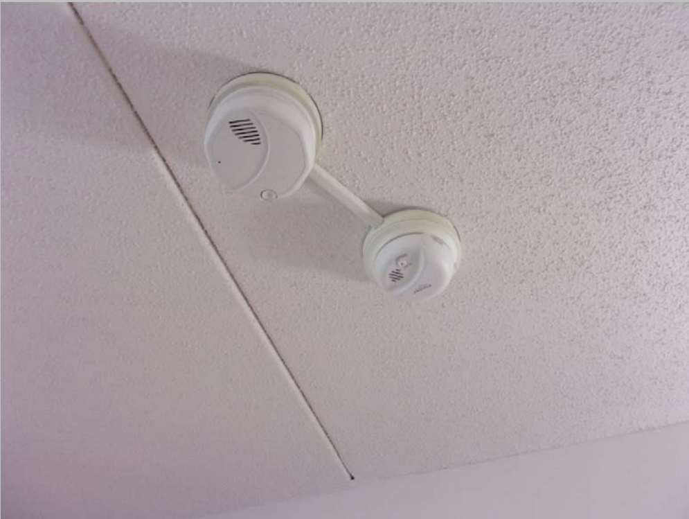
Dwelling unit hardwired smoke and carbon monoxide detectors
