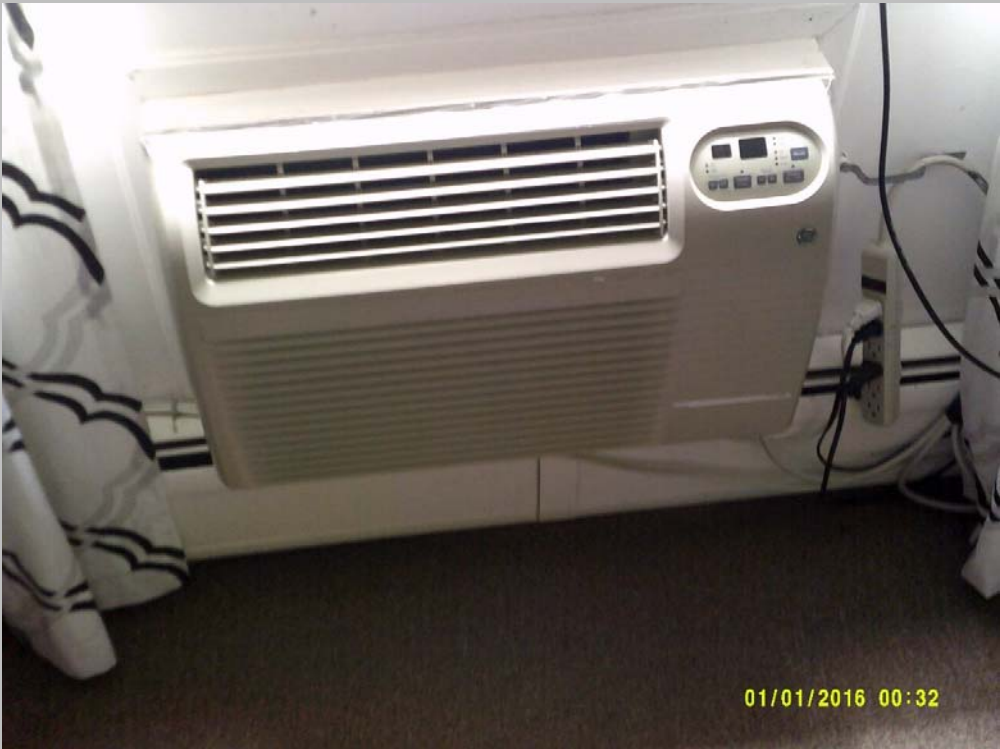
Dwelling unit thru-wall air conditioning unit
