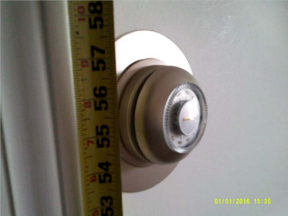
Dwelling unit thermostat mounted above 48" (Critical Repair)
