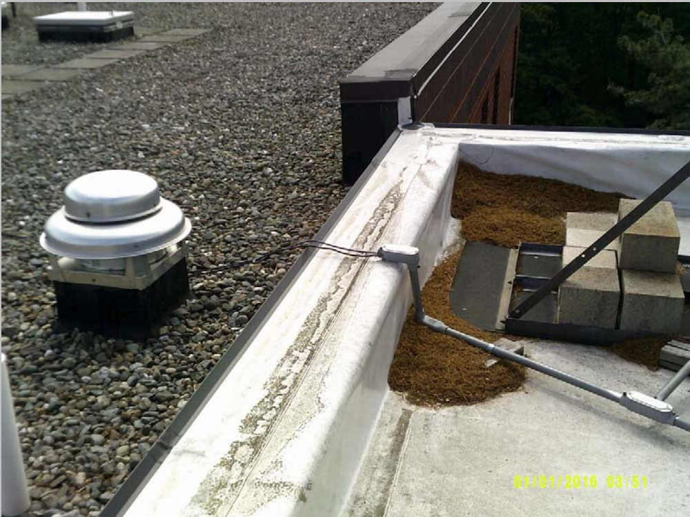
Coleman House I roof with tree debris (Non-Critical Repair)
