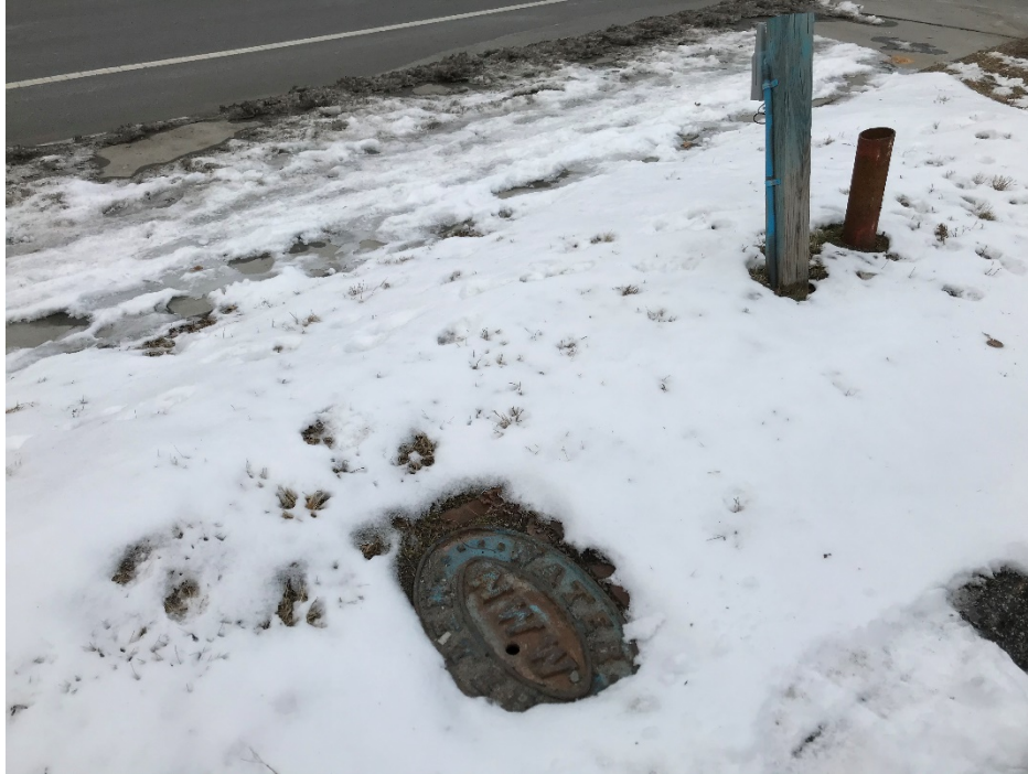
Water Meter Pit within grass strip along driveway
