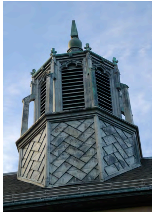
Figure 4: Close-up view of cupola.
