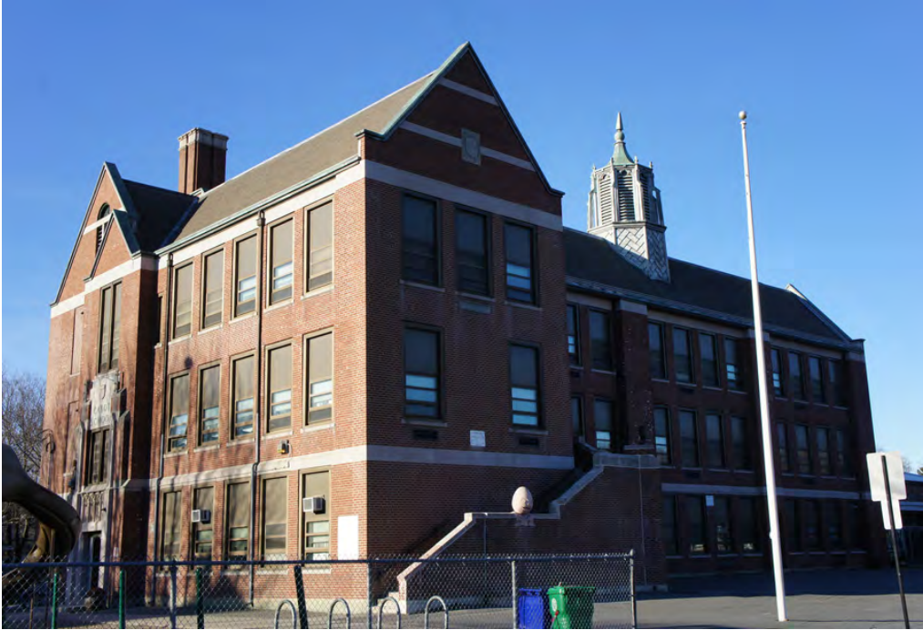
Figure 2: The tall windows set in a simple rhythm around the perimeter of the building were designed to provide daylight deep into the building. This function, as well as the aesthetic character of the building, was greatly affected by the installation of inappropriately designed replacement windows.
