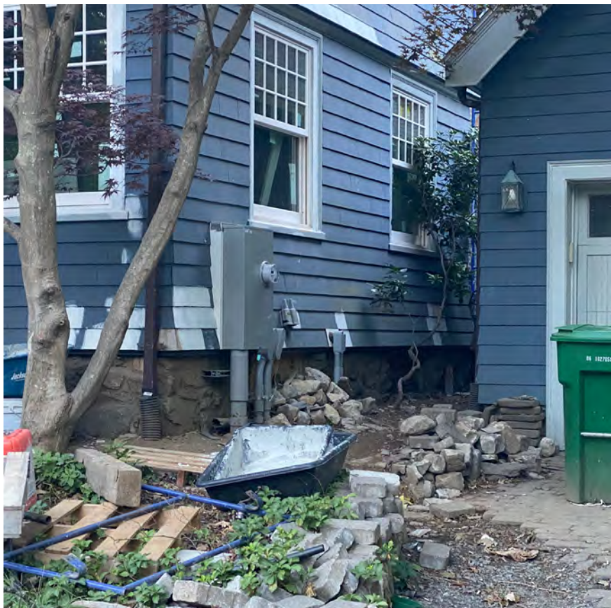
New Electrical Box (Same Location) Unpainted
