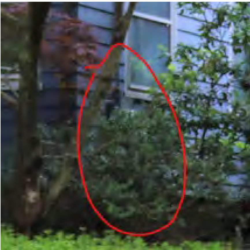
Existing Electrical Box
