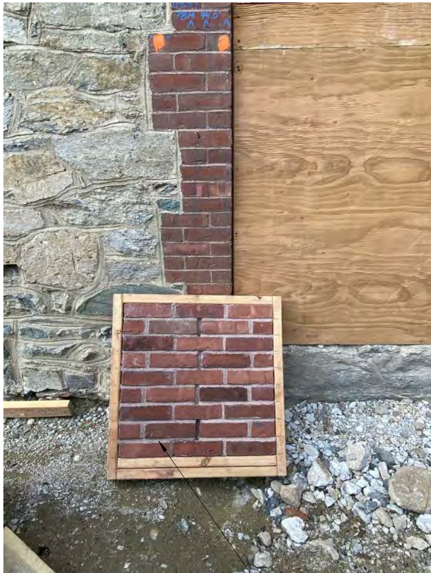
THE MORTAR COLOR ON THE LEFT SIDE OF THE MOCK UP WAS CHOSEN
