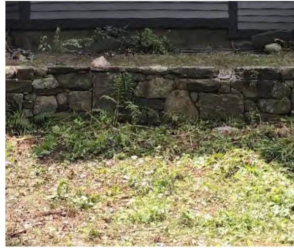
Existing retaining wall to remain. Use existing wall as inspiration for new retaining walls.
