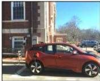
Clean vehicles: City Hall EV charging station
