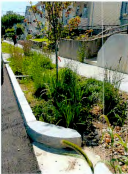
Bioretention Curb Bump-out Edenfield Ave, Watertown
