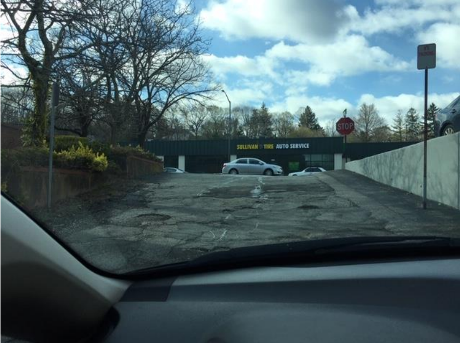
Top of Dunstan Street hill. Shows slope and narrow width of street.
