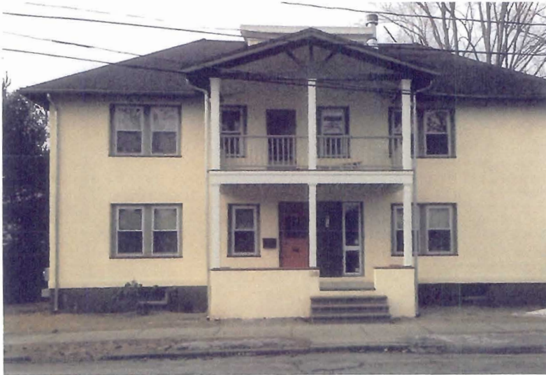
North/Front Elevation Masonry restoration. Rebuild existing dormer. Relocate DU1 entry to side.
