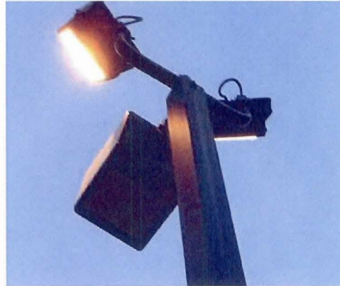
(Pole Mounted Flood Lights)
