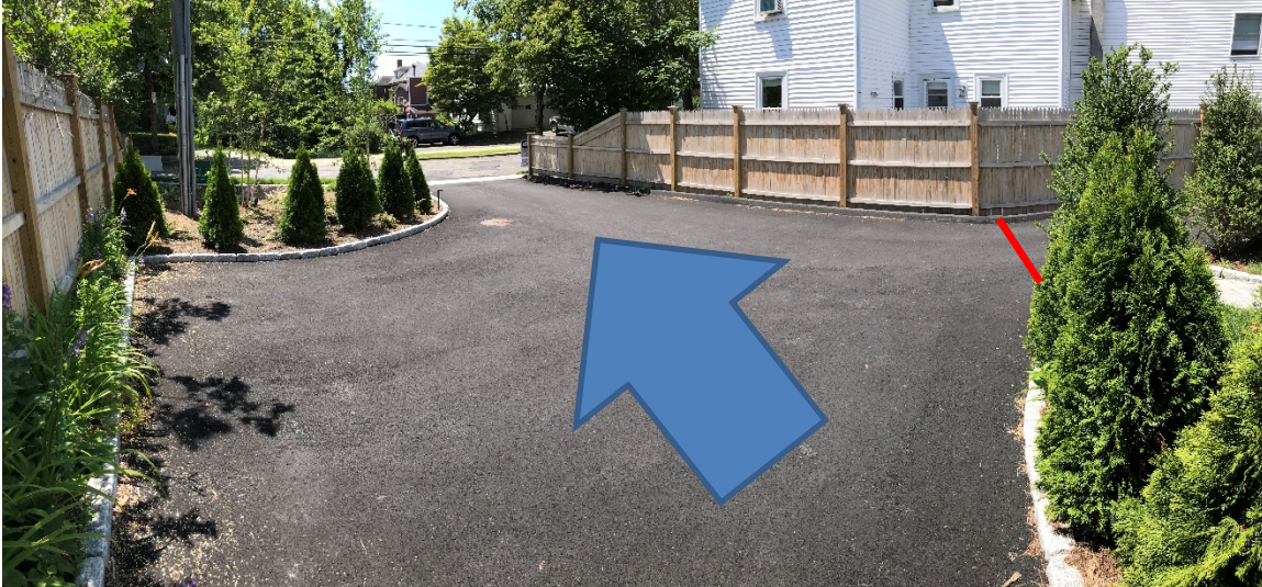
This portion of the driveway is uncontrolled runoff towards Beecher Place
