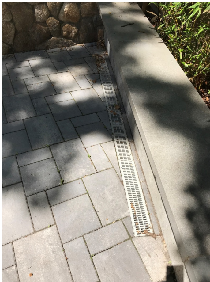
This area drain was not accounted for in the original drainage calculations
