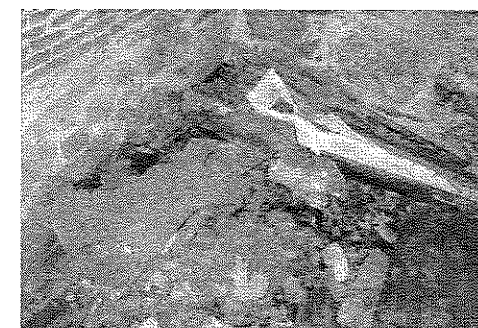
Top: The Fuller-Hull Tomb before emergency restoration work. Middle and Bottom: Interior views of the vault.
