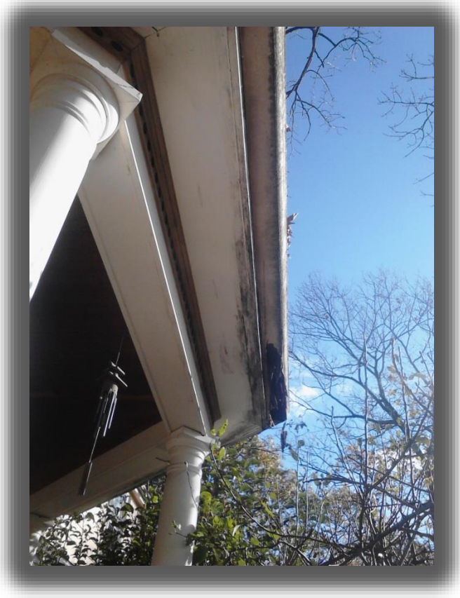
7 Year Old Wood Gutter -Arlington, MA
