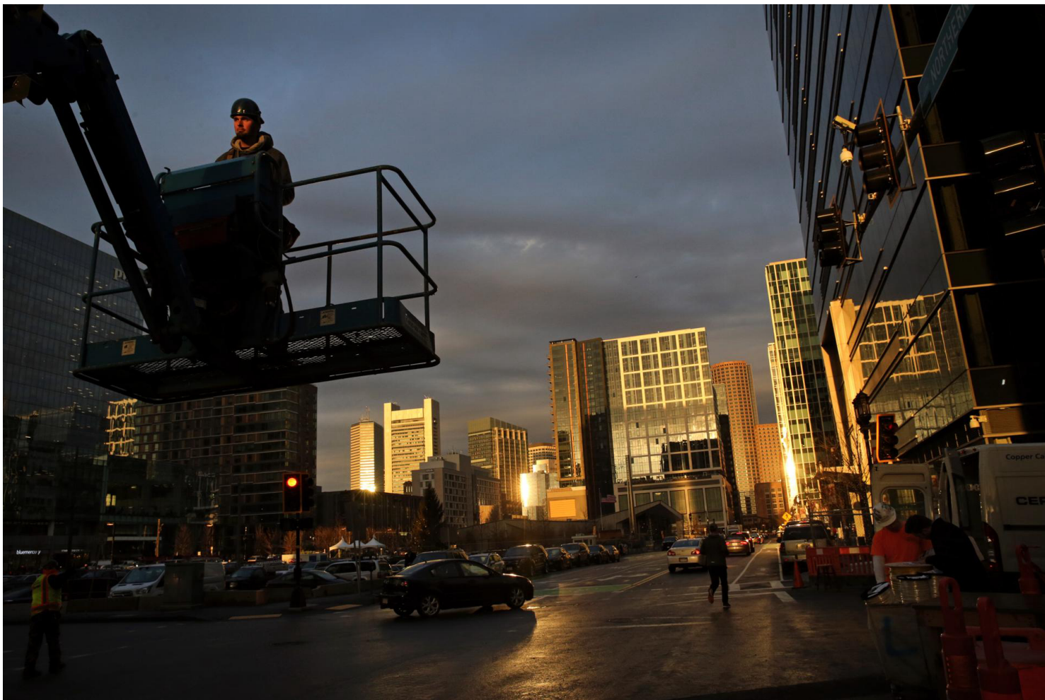
The Seaport's building boom continued at Pier 4 on Northern Avenue. Construction workers have logged nearly 9 million work hours since 2006, according to a Globe analysis of data collected by the city. (Craig F. Walker/Globe Staff)
