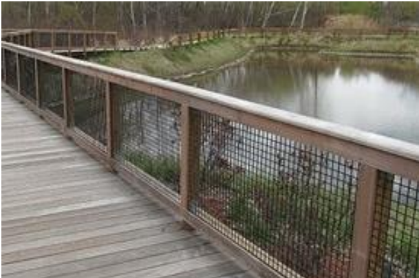
Cantilevered Deck Safety Railing
