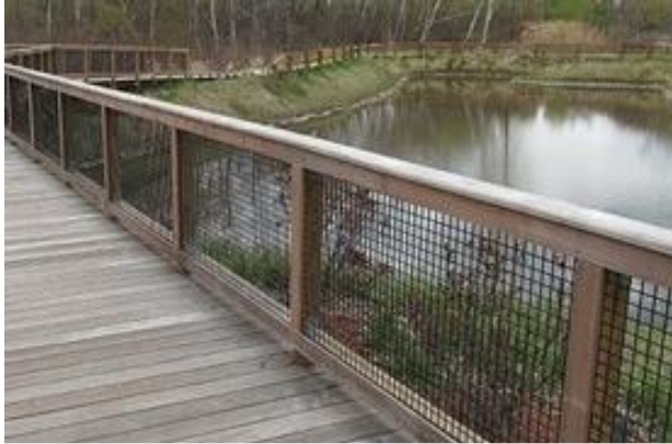
CANTILEVERED DECK SAFETY RAILING
