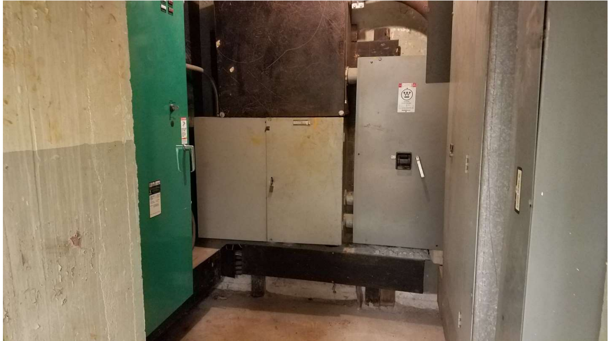
This space is extremely small and does not meet current electrical code requirements.
