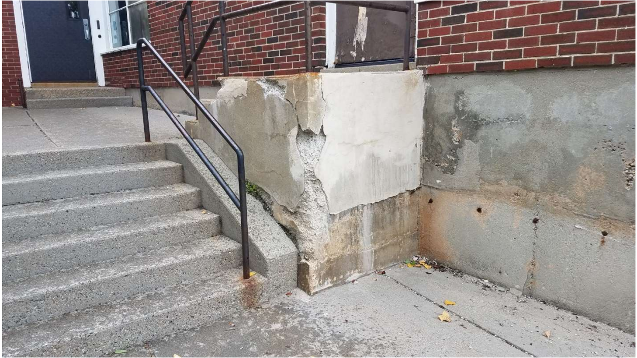
Repairs have been made to this many times before, but clearly more work is needed.
