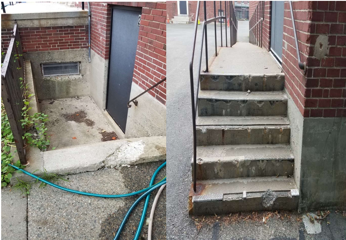
Modest repairs are needed before these become larger replacement projects.
